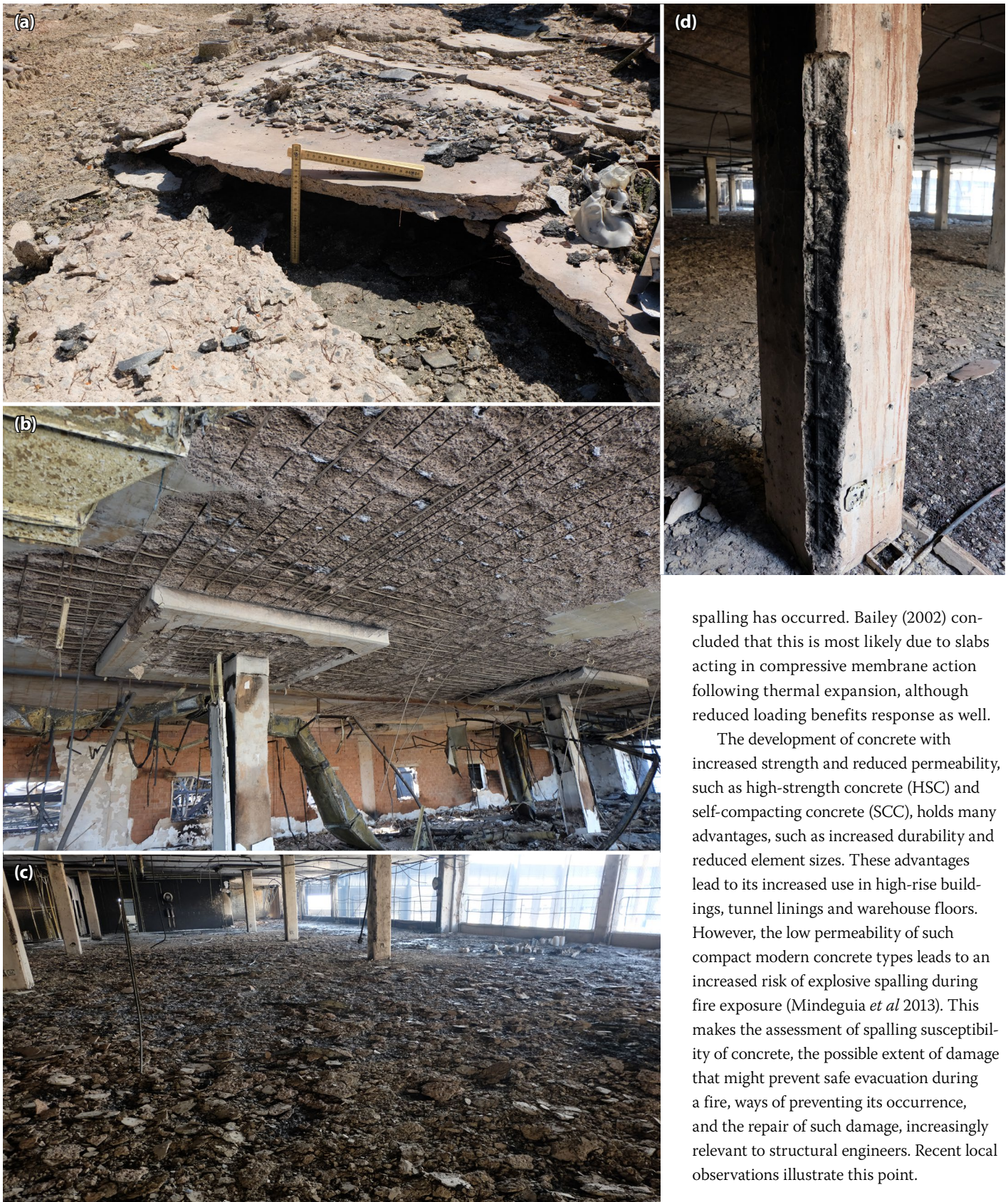
Figure 1 Examples of recent fire-induced spalling damage during a fire damage assessment by the author following the July 2021 riots in South Africa: (a) explosive spalling of the steel-fibre-reinforced concrete floor, (b) spalling to the soffit and drop panel of an office building, (c) spalling to the top of an exposed slab, and (d) corner spalling of a column
