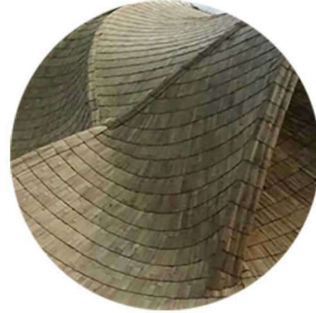
3// SECONDARY ROOF STRUCTURE bamboo roof shell truss structure with bamboo roof skin
