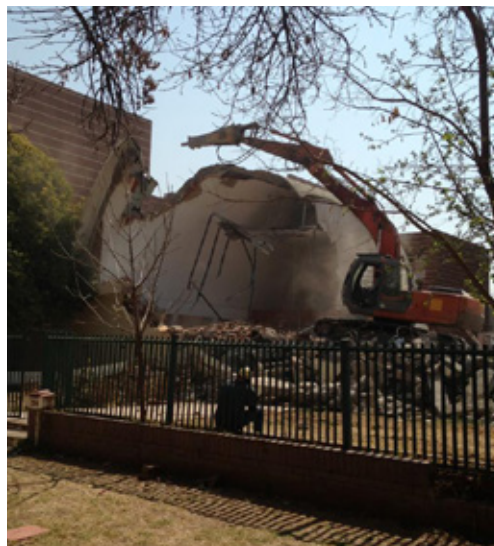
Figure 10 Roberts and Cassells ca 1959. The Chapel of the CLDS as viewed from Zastron Street during demolition. (photo: H. Lampbrechts, August 2013).
