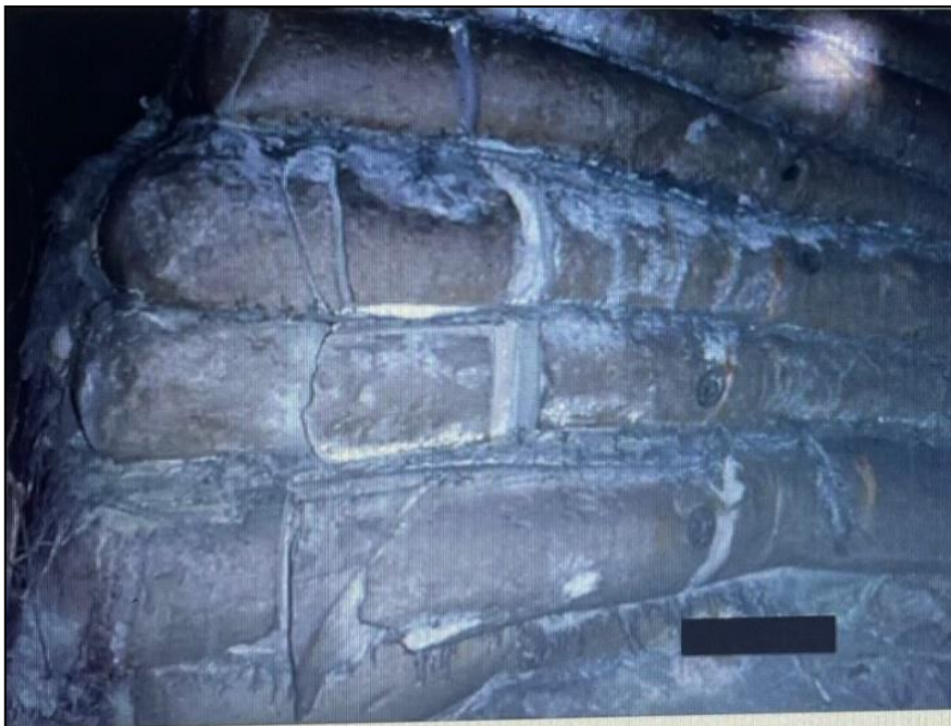
Figure 2-47. Condition of the grout packs adjacent to a mined-out pillar (D. F. Malan 2023, pers. comm.).
