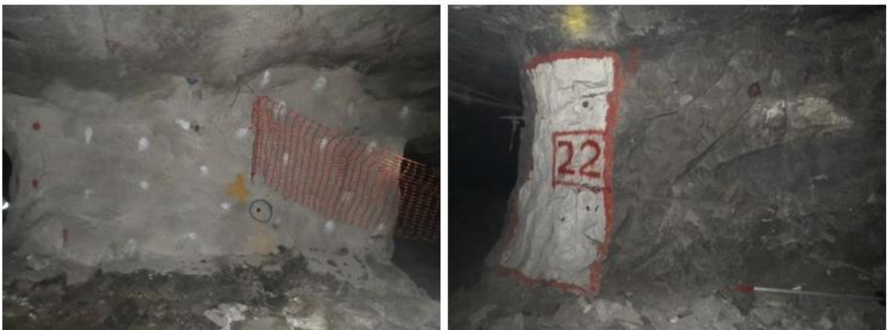
Figure 5-3. Condition of a rehabilitated pillar (left) compared to most of the pillars in the area of interest (right) (courtesy of D. F. Malan).
