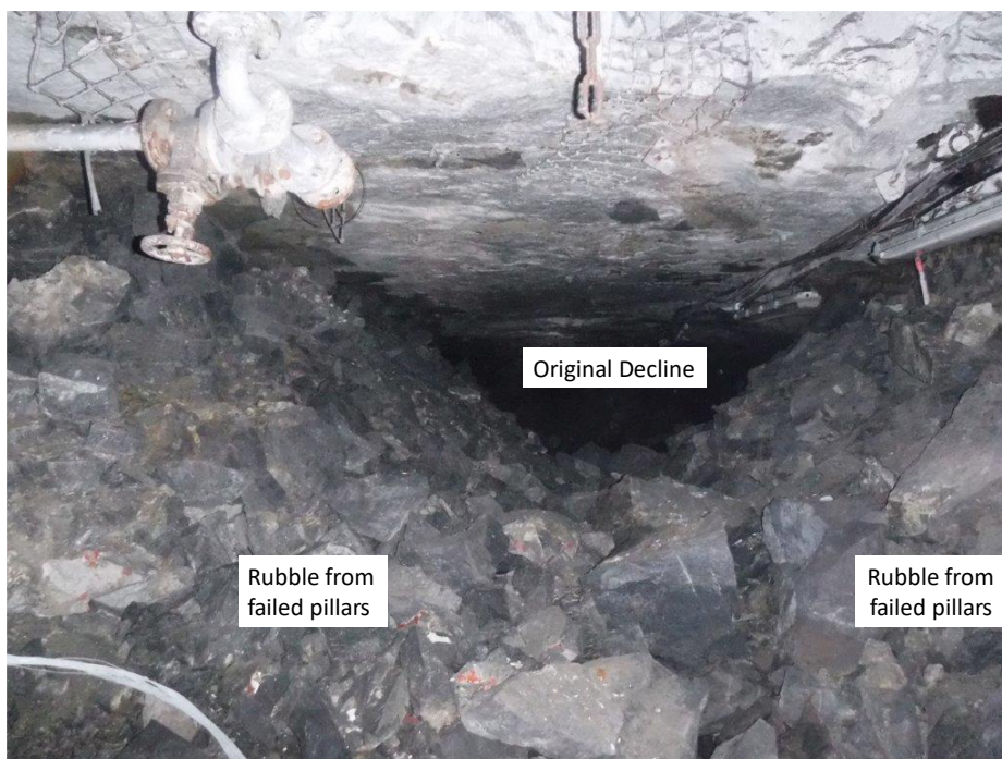
Figure 2-14. Some of the pillars were completely crushed during the collapse. This expansion of the pillars could have been arrested by using backfill (after Couto and Malan, 2023).
