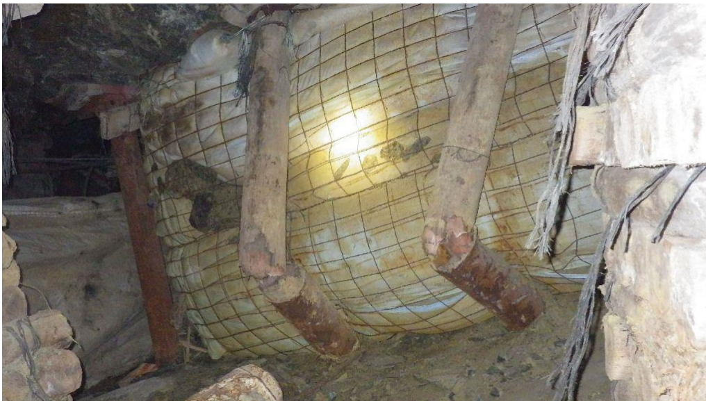
Figure 2-21. A backfill paddock in a deep tabular gold mine (courtesy of D. F. Malan).
