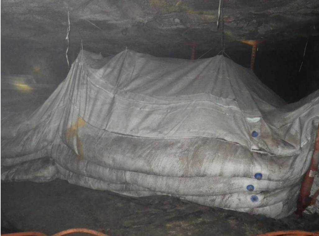
Figure 5-14. Use of backfill bags in an attempt to seal the holing between adjacent pillars (courtesy of D. F. Malan).
