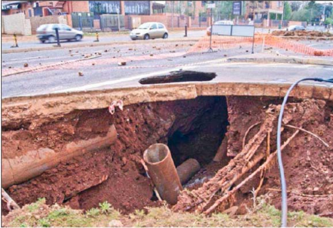
Fig. 6. A sinkhole that occurred in Jean Avenue in Centurion, South Africa, in 2012, removing part of a road. (Oosthuizen and Van Rooy, 2015).
