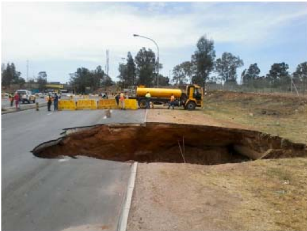
Fig. 7. A sinkhole in Benoni, Gauteng, RSA that led to a road closure in 2019 (City of Ekurhuleni, 2019).
