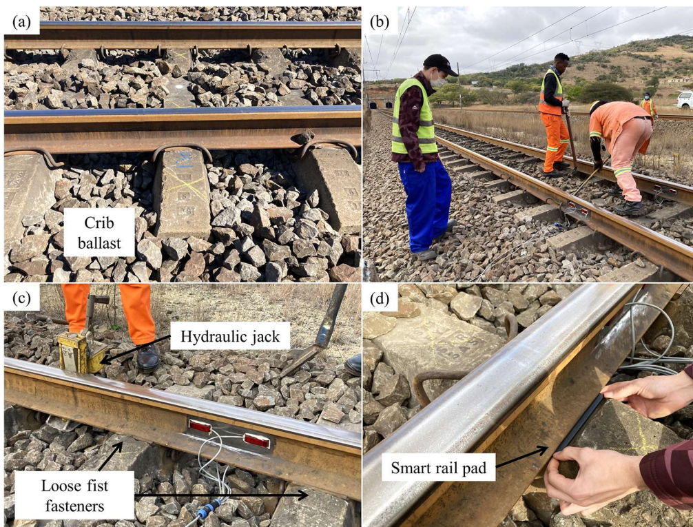
Figure 8: Rail pad replacement: (a) opening made for removing Fist fasteners, (b) process of removing Fist fasteners, (c) hydraulic jack to lift the rail and (d) the installation of the smart rail pad
