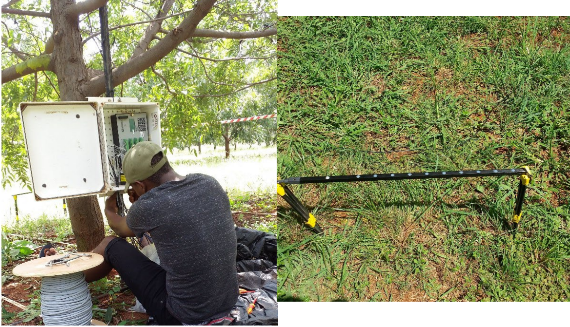
Figure 3.4 Installation of quantum sensors in the orchards, as well as wiring the CR3000 datalogger.
