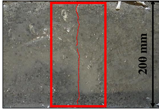
Figure D.2: Final crack width for ERS-2, indicated in red
