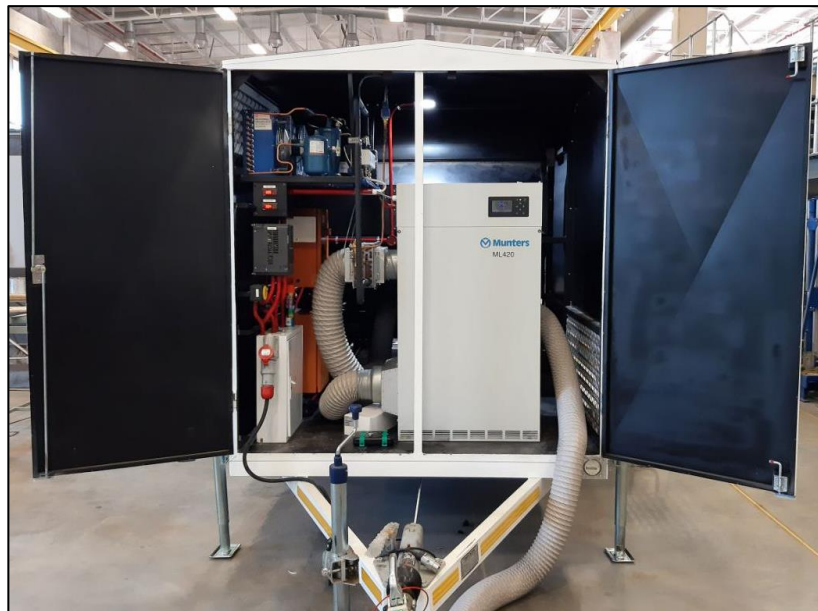
Figure 5-8: Control room of the MCC
