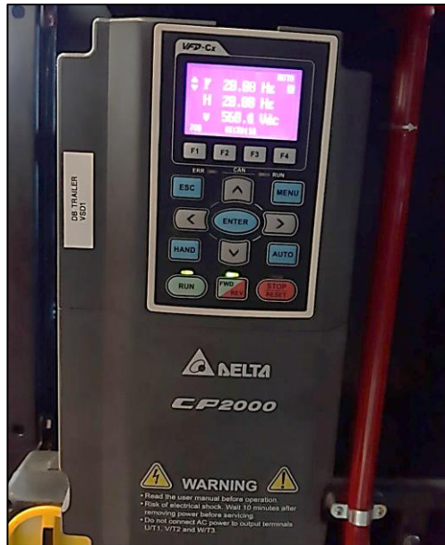
Figure 5-10: DELTA CP2000 variable speed drive
