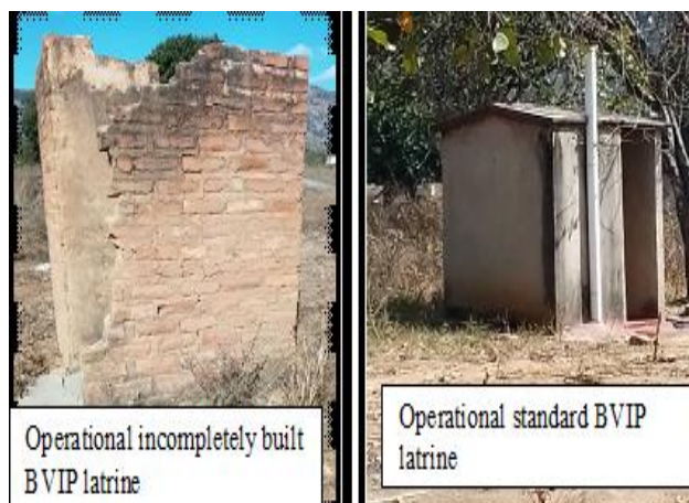
Fig. 1 Latrines in a rural district of Zimbabwe
