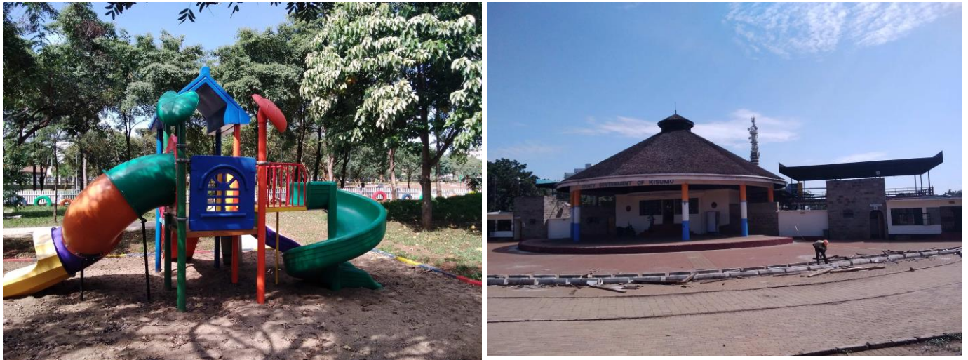
Plate 4.4: a) Children play area, b) On going drainage works at Jaramogi Odinga Odinga Sports Ground. Source: Author, July 2021
