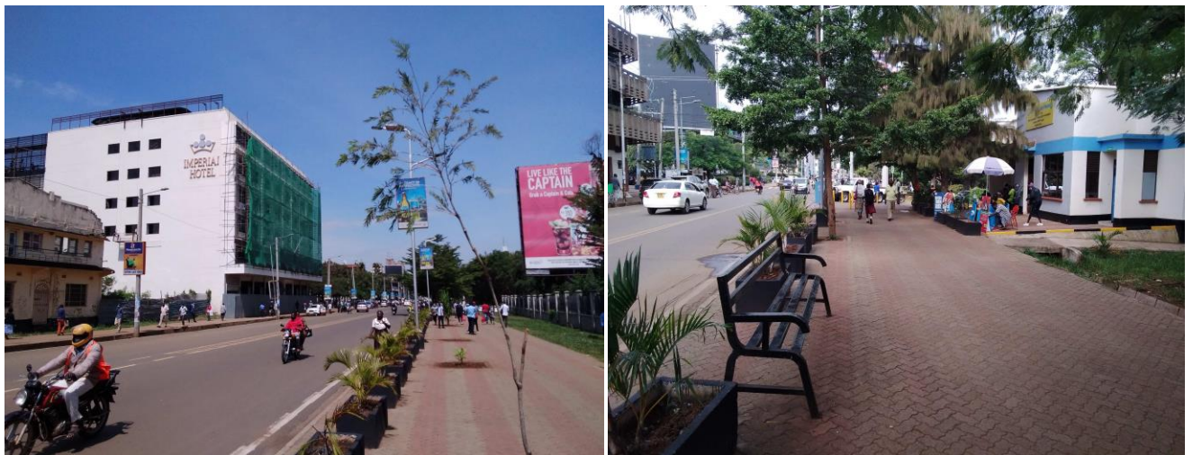
Plate 4.2: Installed concrete planters along Jomo Kenyatta Highway within cabro paved pedestrian walkway with a green strip along the wall fence for Jaramogi Oginga Sports Ground. Street seats are provided for relaxation.
