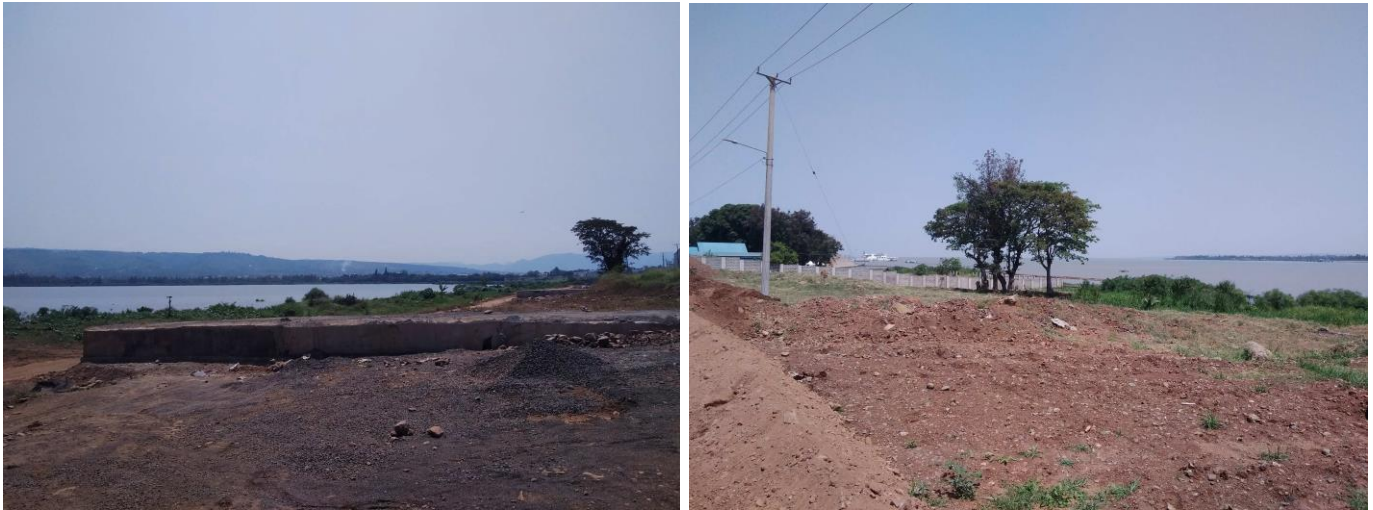
Plate 4.19: The Lakefront after demolition of informal hotel structures b) Part of the revamped Kisumu Port
