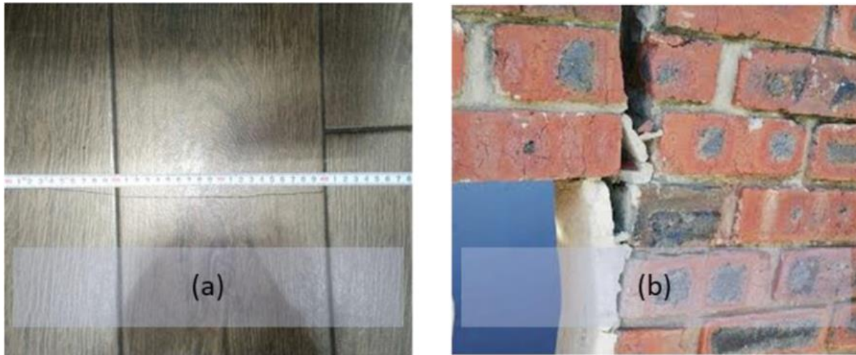
Figure 3.2 Structural damage resulting from the 6 February 2016 KwaZulu-Natal offshore earthquake (a) Long hairline crack at the Vodacom store, Hammarsdale mall, (b) Damage to a government subsidised Reconstruction and Development Programme (RDP) home in Hammarsdale
