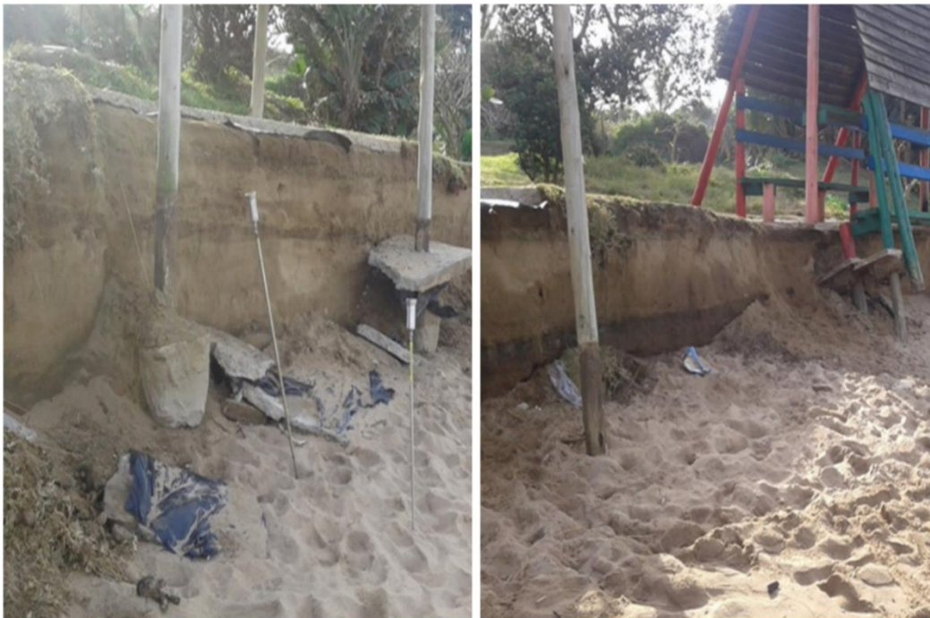
Figure 4.2 Damage caused by the disturbance in the tides after the Sundumbili 16 June 2015 earthquake (courtesy of Sanele Mkhwanazi).
