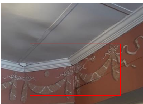
Figure 53: Previous damage from a leak.
