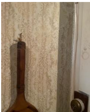
Figure 77: Damage from a previous leak in the boy's bedroom.
