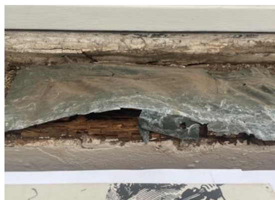
Figure 18: Rotting wood in the conservatory.
