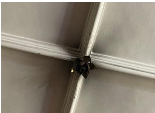
Figure 11: Blackening of paint from an electrical shortage, seen in the dining room (ground floor).
