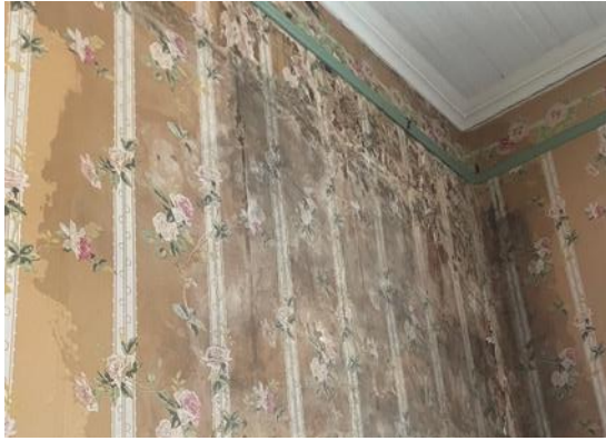
Figure 25: This image is after cleaning, in August 2022. The damage and loss of material due to the mould, as well as cleaning process, is extensive.
