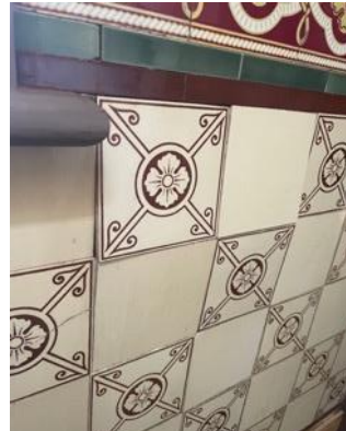
Figure 2: Kitchen tiles lifting off the wall from movement of house.
