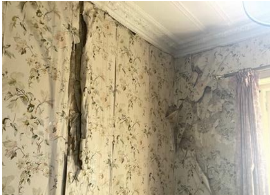
Figure 13: Peeling wallpaper and molding of ceiling in the dressing room (first floor).
