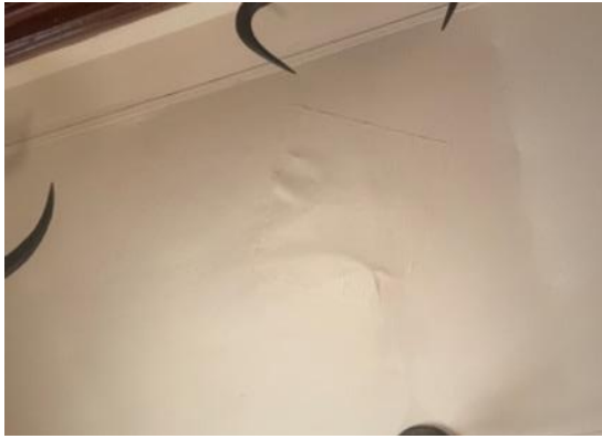
Figure 25: An example of where the ceiling has been patched-up following damage from a leak.
