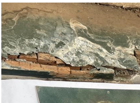
Figure 17: Water damage in the conservatory. Tidemarks Visible showing where water has previously pooled.
