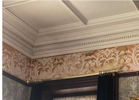
Figure 14: Water damage seen on wallpaper in dining room (ground floor).
