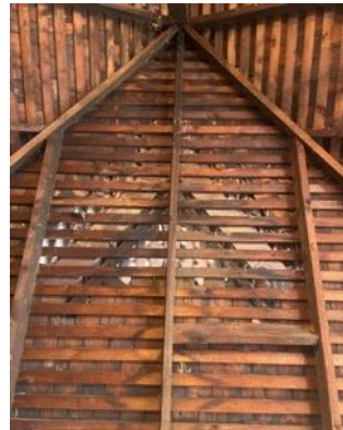
Figure 28: The roof in the servant's hall has no ceiling.
