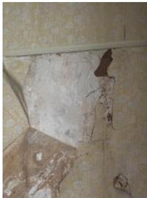
Figure 15: Peeling wallpaper in the yellow bedroom. The wall is waterlogged which resulted in the failure of the wallpaper adhesive.
