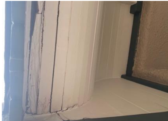
Figure 20: Degradation of awning wood as a result of water damage from rain.
