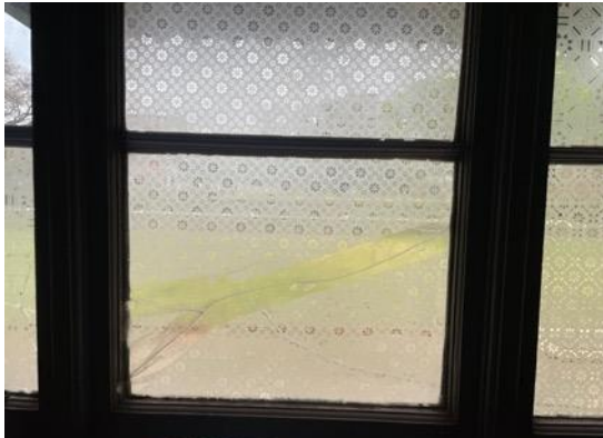
Figure 1: A cracked window in the kitchen resulting from the sinking movement of the house.
