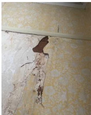
Figure 3: An example of a waterlogged wall, seen here in the yellow bedroom (first floor).
