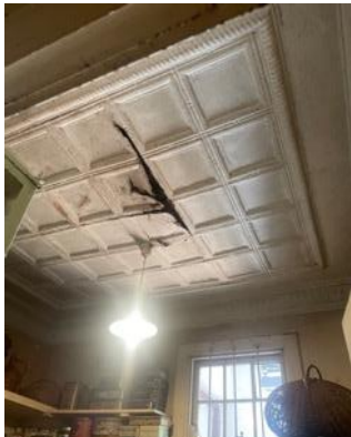
Figure 87: The pantry roof is in very poor condition as a result of the geyser leak and has corroded in some areas.
