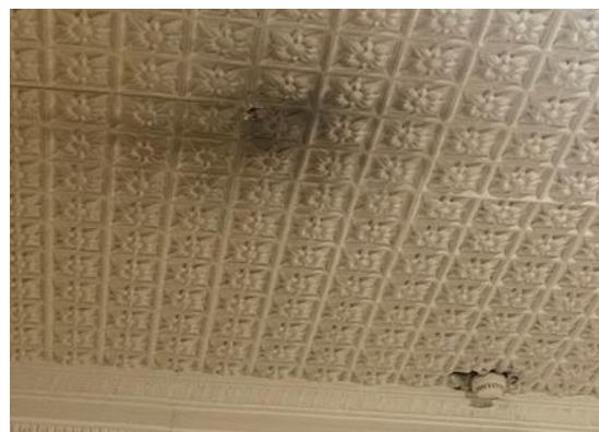
Figure 12: Blackening of paint from an electrical shortage, seen in the exhibition room (ground floor). A fire alarm can be seen in the bottom right of the picture.
