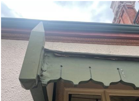
Figure 21: Water damage to wooden awning.
