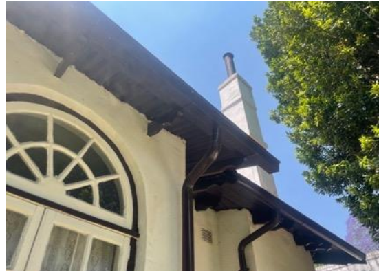
Figure 38: The roof is well maintained and the eaves are free from debris.
