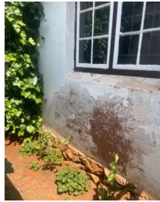
Figure 140: Paint is peeling under the left window of the servant's hall.
