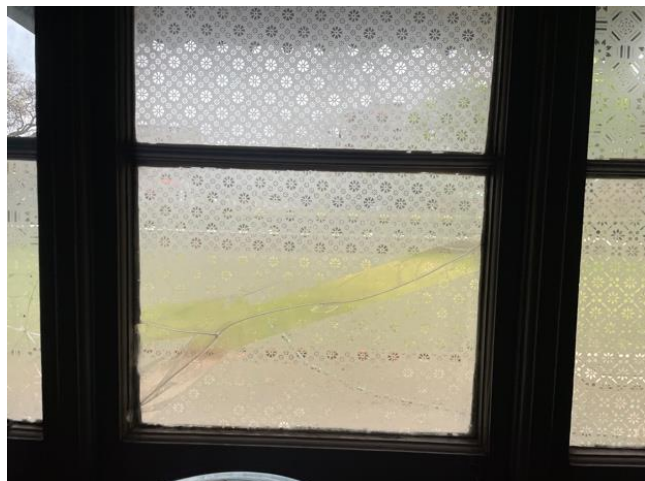
Figure 3: A crack in the southside kitchen window as a result of the pressure of the sinking building.
