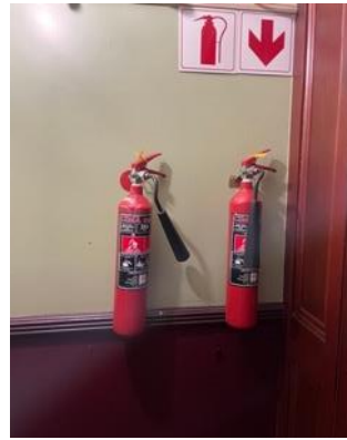
Figure 10: Fire extinguishers and signage on the ground floor, located next to the billiards room.
