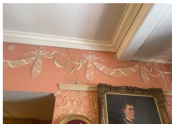
Figure 54: Some cracking of the wall.
