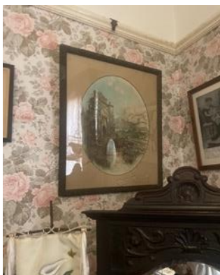
Figure 131: Picture with previous water damage.
