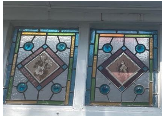
Figure 28: Fading of colours on windows due to UV exposure, as seen in the conservatory.
