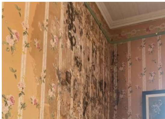
Figure 24: Mould on the wall in the nursery in March of 2022 as a result of the damp in the wall. .
