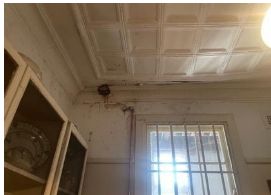
Figure 84: Damage to wall and ceiling in the butler's pantry from a leaking gas geyser that was removed. The ceiling now bulges down.
