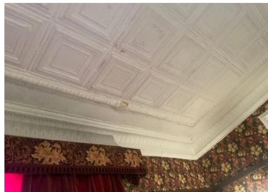
Figure 96: Damage on the roof from a leak in the library.
