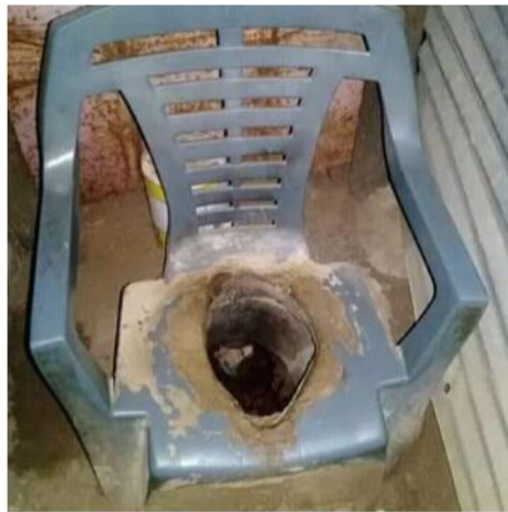
Poor ablution facilities (Photo by P24)
