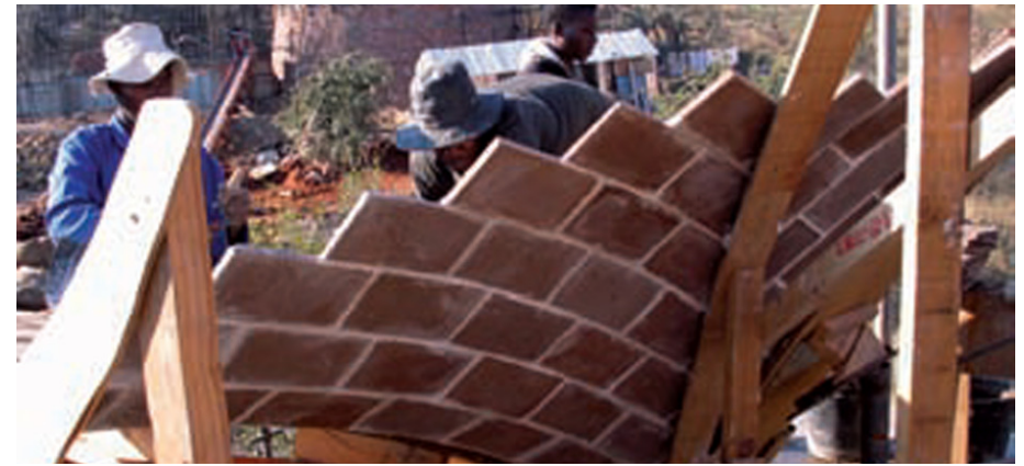
Figure 84 _ The construction of the vaults at the Mapungubwe Interpretation Centre (Ramage et al, 2008)
