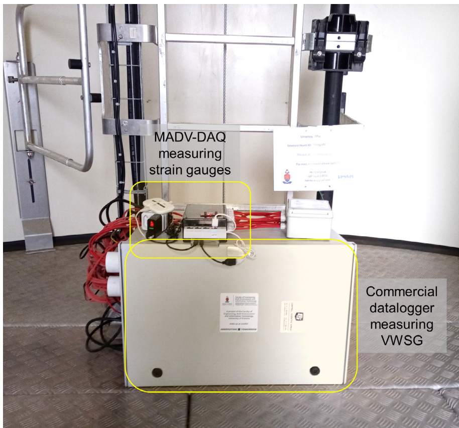
Fig. 12. MADV-DAQ and commercial datalogger installed inside the wind turbine tower.
