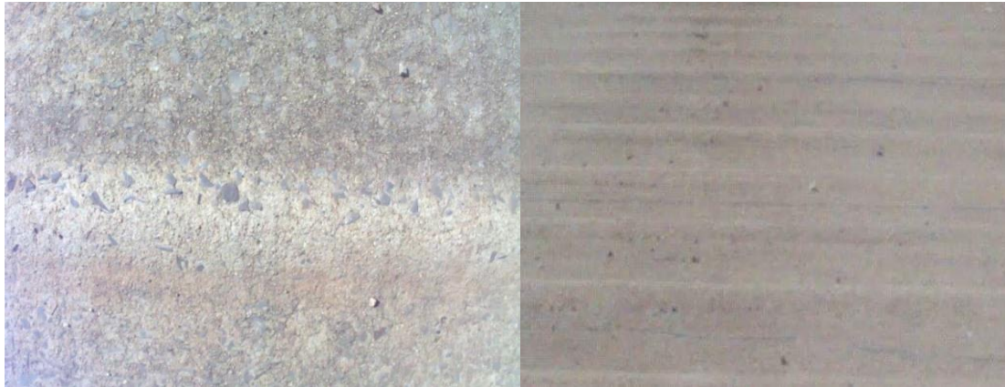
Figure 4.15: Angled corrugation road profile of downward- and forward-facing camera data
