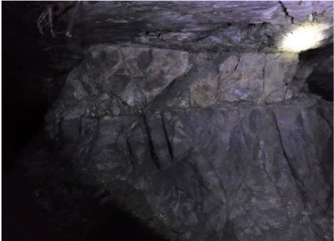
Figure 4-6. The typical condition of a pillar in the Level 2 failure zone.
