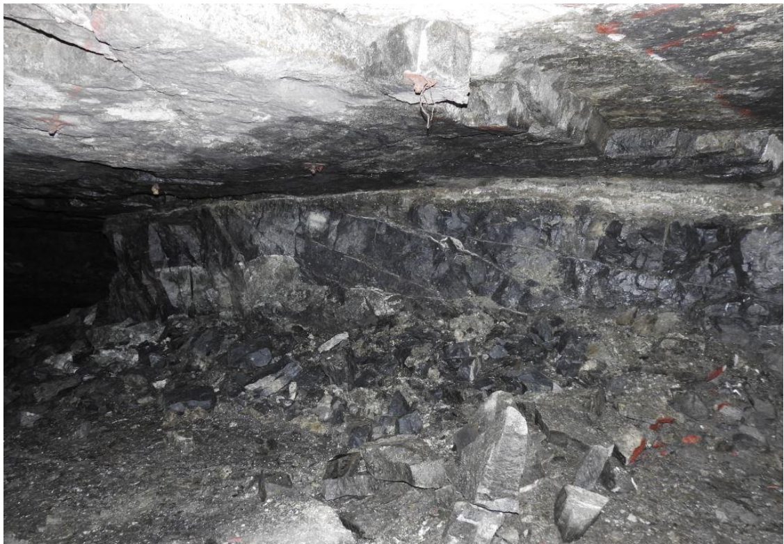
Figure 4-11. Failure of a pillar as a result of the presence of jointing in the Level 2 failure zone.
