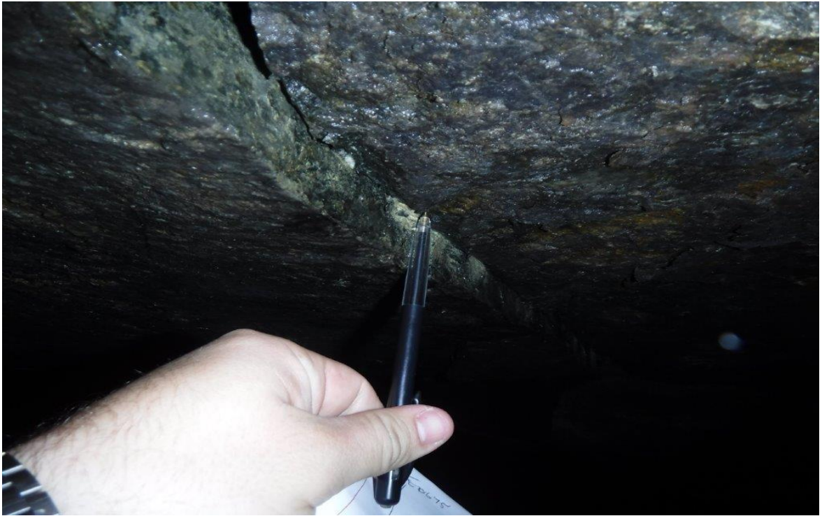
Figure 4-20. Relative displacement of a tensile crack in the Level 5 failure zone close to the Decline position.
