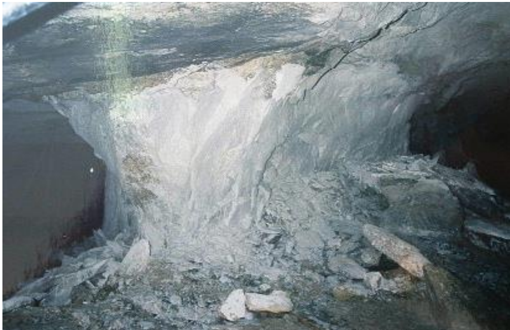
Figure 2-11. An example of pillar scaling in areas where there is a “frozen” interface between the pillar and the hangingwall. The typical “hour-glass” failure mode is evident (photograph courtesy F. Malan).
