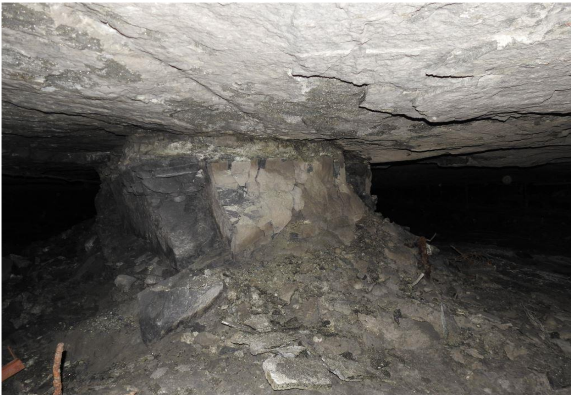
Figure 4-13. Extensive scaling of a pillar in the Level 3 failure zone. Note the hangingwall deterioration due to significant closure occurring.
