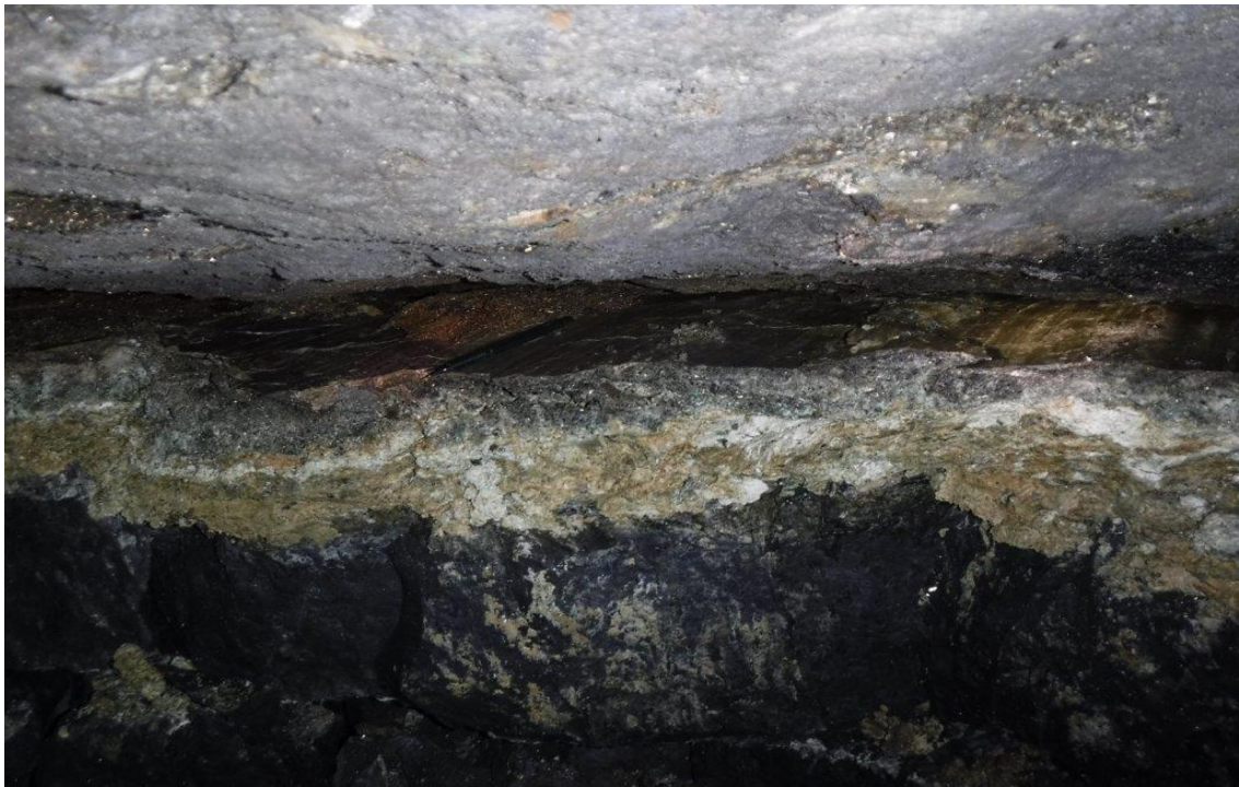
Figure 4-17. A close-up photograph of the alteration zone in the Level 4 failure zone. It is wet and it has evidence of slickenside surfaces. There is a gap between the pillar material and the hangingwall in this area.
