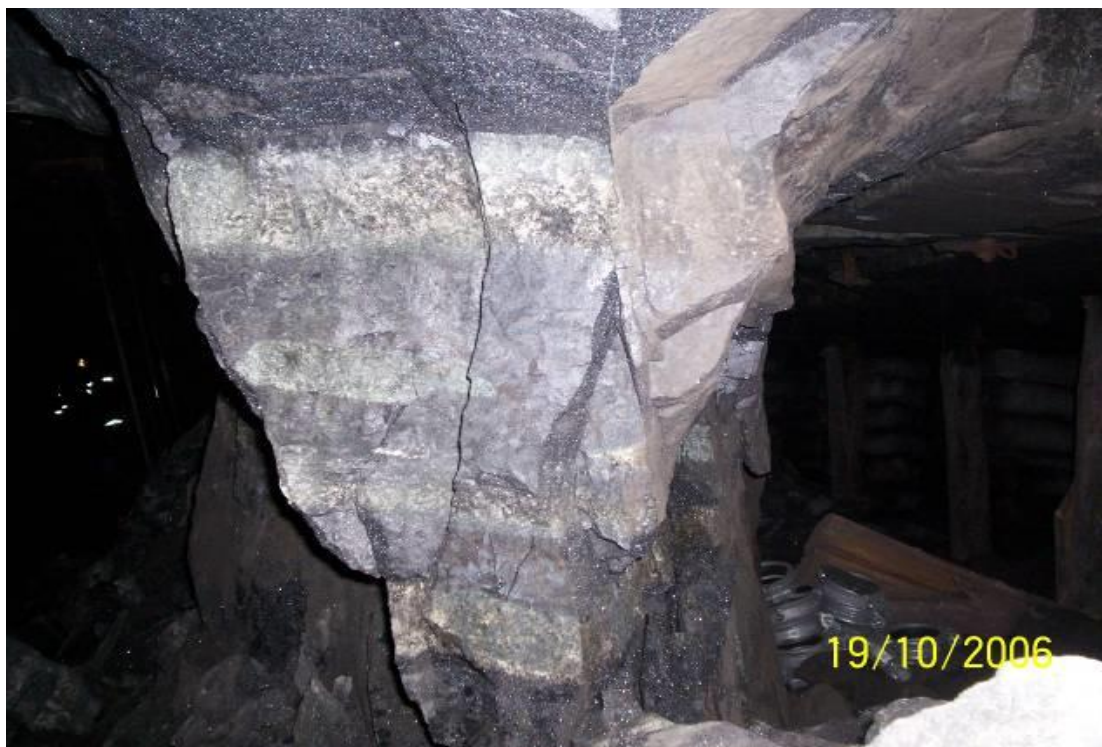
Figure 2-12. An examples of pillar scaling in areas where there is a “frozen” interface between the pillar and the hangingwall at Hossy shaft. Again, this results in the typical “hour-glass” failure mode (photograph courtesy F. Malan).
