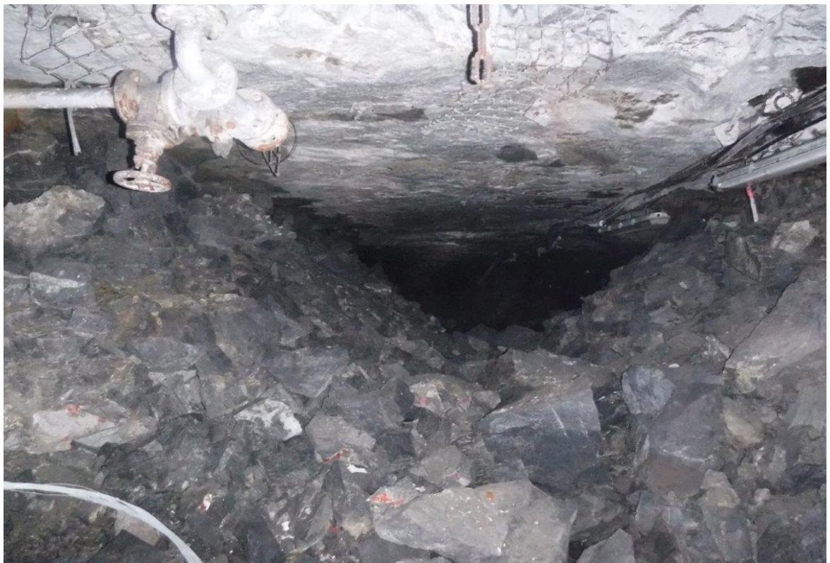
Figure 4-21. A view illustrating that the pillars adjacent to the Decline have been completely crushed.
