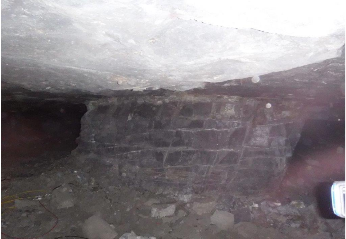
Figure 4-10. A pillar in the Level 2 failure zone with joints and fractures visible.
