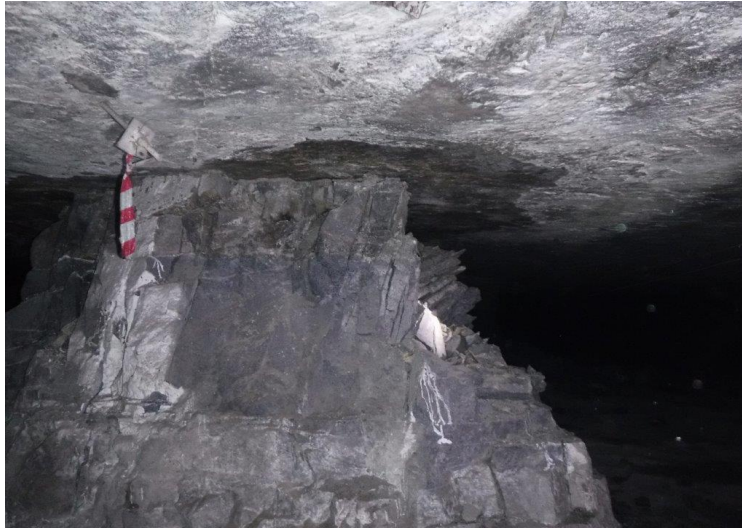
Figure 1-2. Typical pillar failure in areas where weak alteration zones are present.
