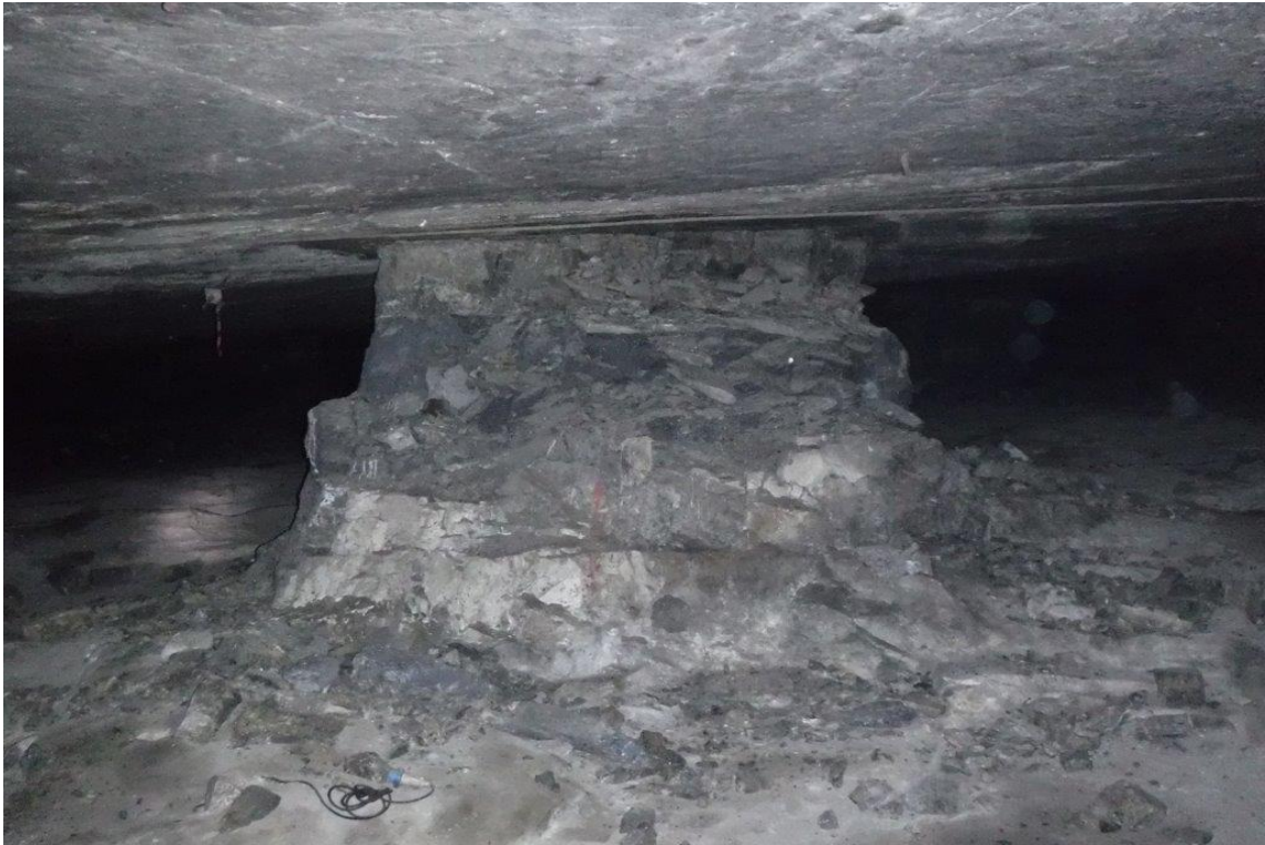
Figure 4-12. A pillar in the Level 3 failure zone showing extensive scaling and failure. The core of this pillar is still deemed to be intact.
