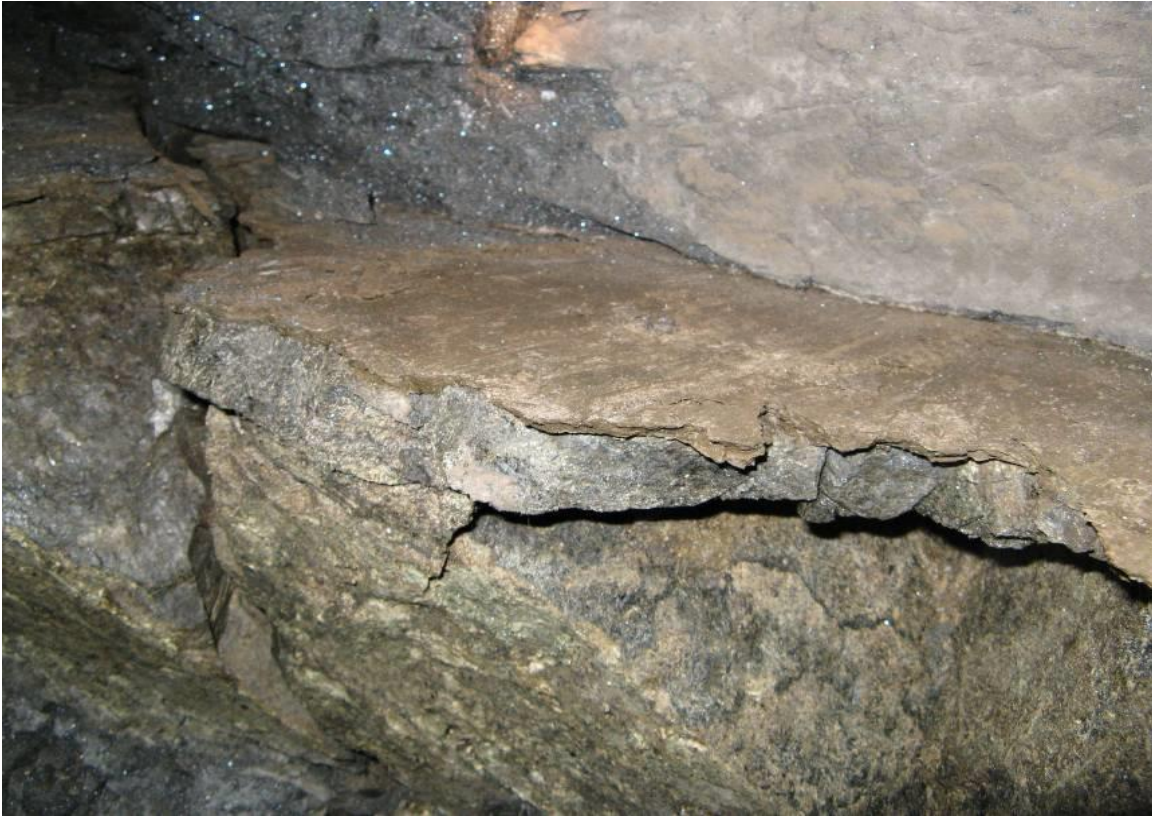
Figure 3-24. Presence of a weak alteration in the pillars at Wonderkop Mine. This photograph clearly illustrates the presence of the clay layer (Malan and Napier, 2011).
