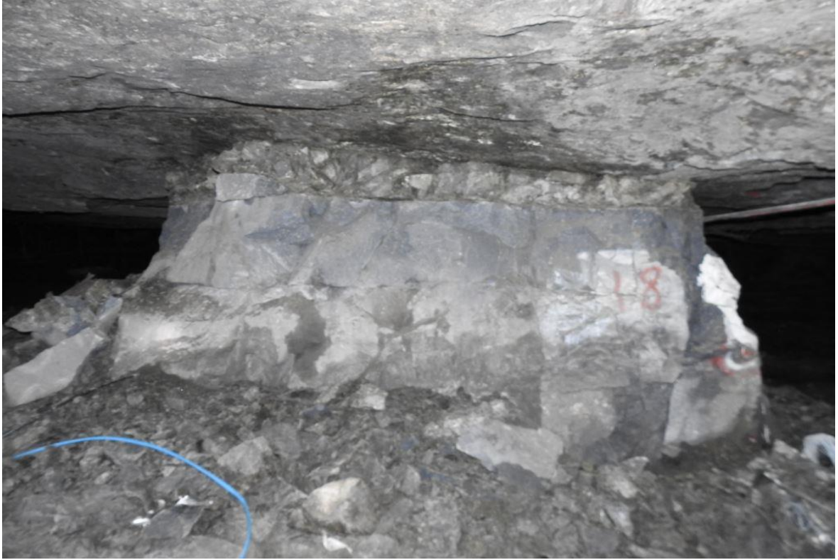
Figure 4-14. A pillar in the Level 3 failure zone with the alteration zone clearly visible.
