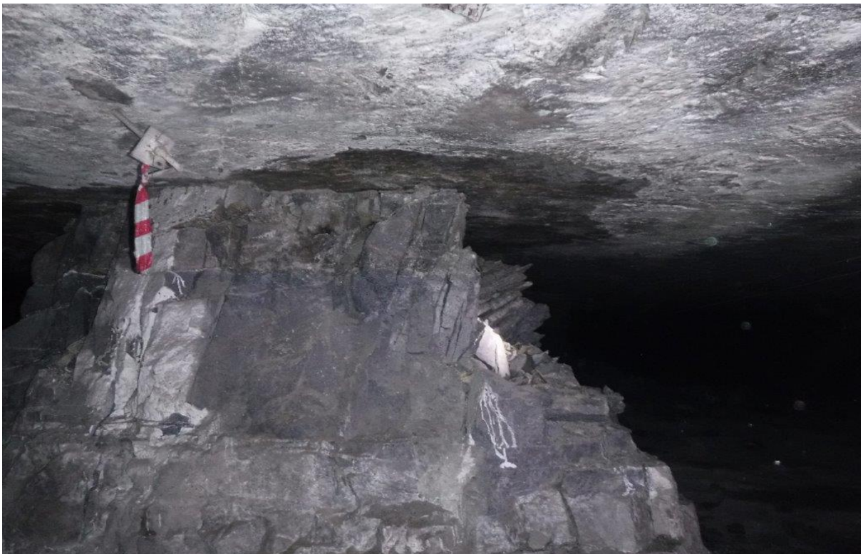
Figure 4-15. A pillar in the Level 3 failure zone where the original size of the pillar is clearly visible on the hangingwall owing to the change in colour caused by the white wash.
