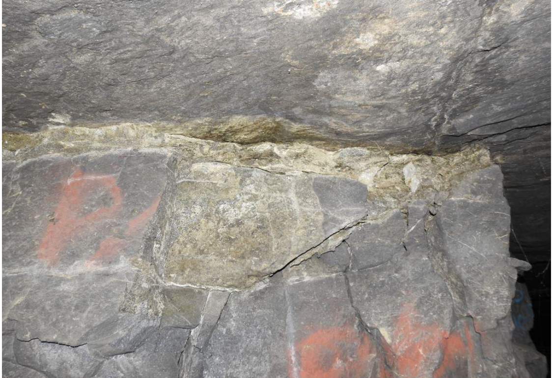
Figure 4-9. Thinning of the alteration zone to approximately 10 cm thick at the top reef contact.
