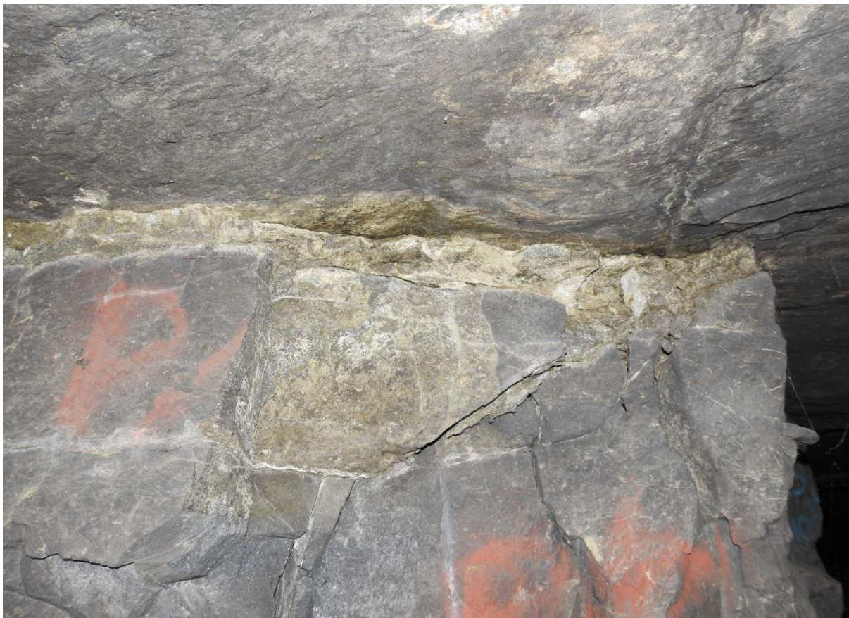
Figure 1-1. A weak alteration layer visible at the contact between the pillar and the hangingwall.
