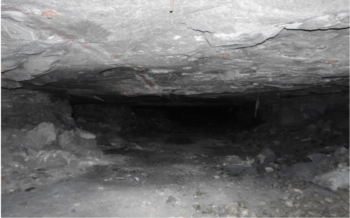
Figure 4-16. Pillar condition in the Level 4 failure zone. The pillars are crushed, but some contact with the hangingwall is still maintained. The large spans indicate that the pillars were not cut to the planned design.
