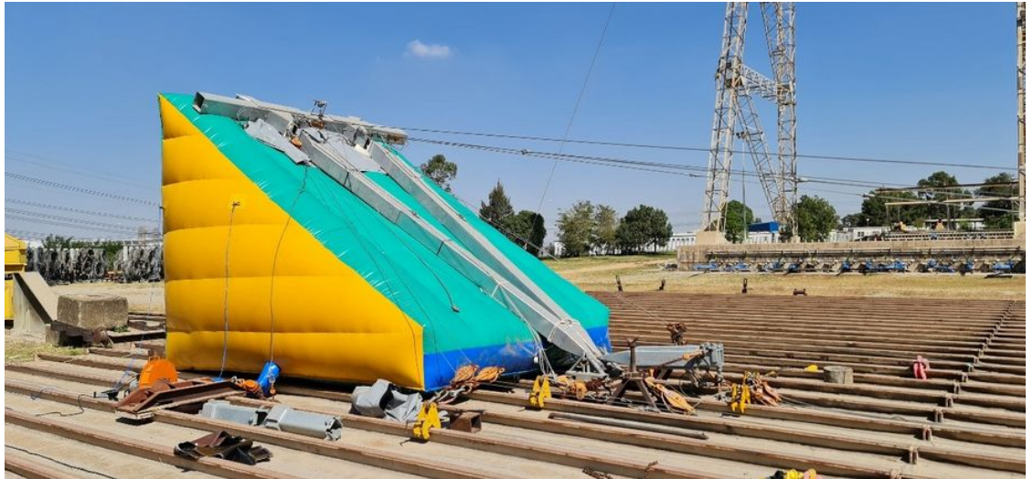
Figure 16 - Use of air cushion to lift model tower – eliminating the gin pole
