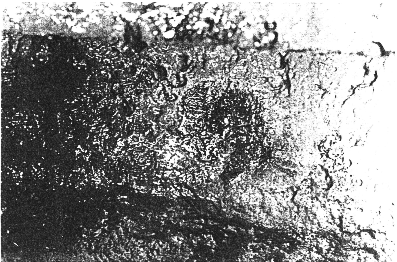
Figure 4.9 : Strainer box at Grootvlei Power Station after three weeks of biodispersant/biocide treatment showing softened nodules on surface (A) and loss of black colouration in underlying pits (B).
