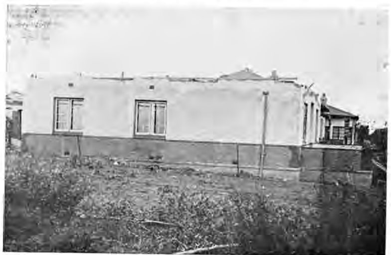
Photograph by Johansons Portrait Studio, Springs. Picture D. Wall plate anchored to top of wall.
