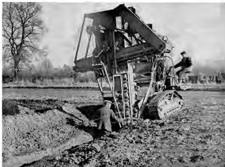
Decentralising London: a trench-digging machine being used in the first stages of the development of Chippingfield, near Harlow. Within the next 20 years an area of 6,300 acres is expected to house 60,000 present day residents of London's northern and north-eastern suburbs.
