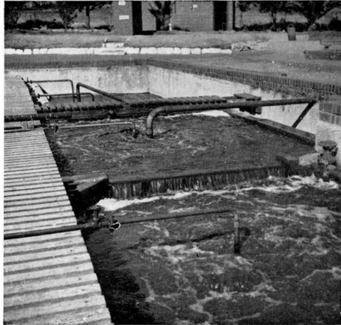
OVERFLOW WEIR IN REAERATION TANK.
