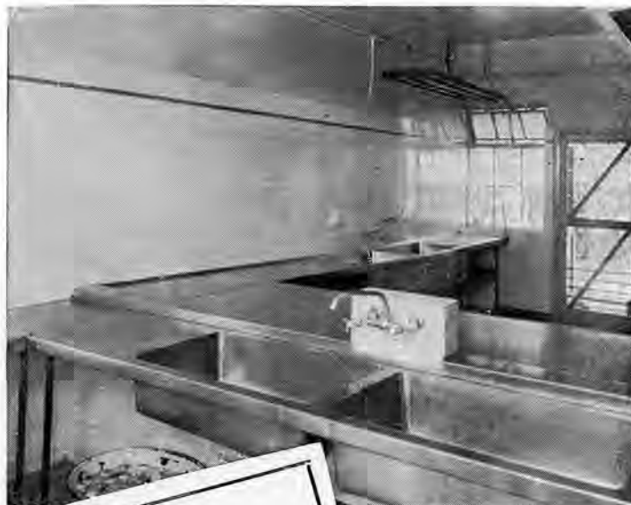
Showing a section of the complete Stainless Steel Kitchen installed by us at the Hotel Cecil, Newlands, Cape.
