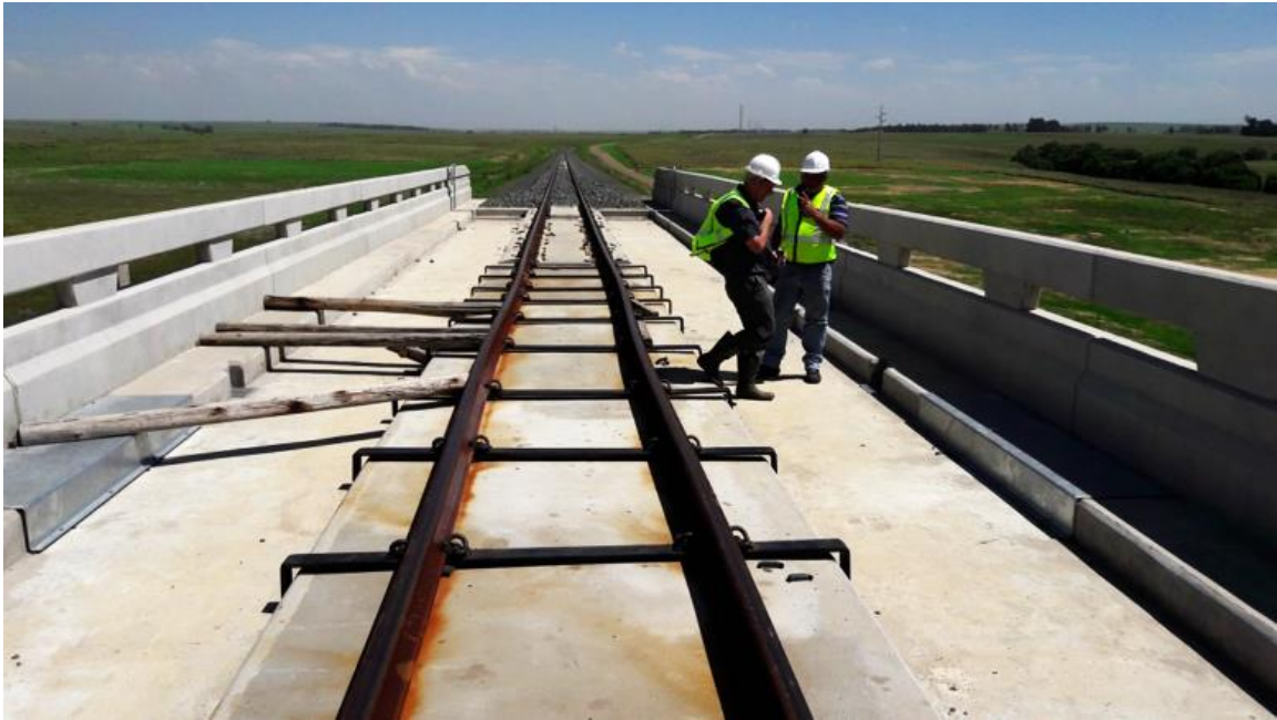
Figure 5.17: Lateral Buckling during Permanent Way Construction (prior to REJ installation)
