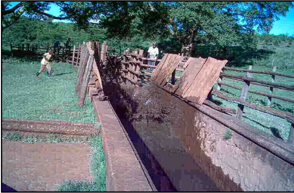
Figure 6.8 The physical condition of the Tshivhulani dip tank
