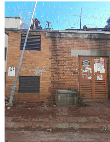
There are however, numerous instances of heritage elements in the process of deterioration and dereliction, largely due to neglect
