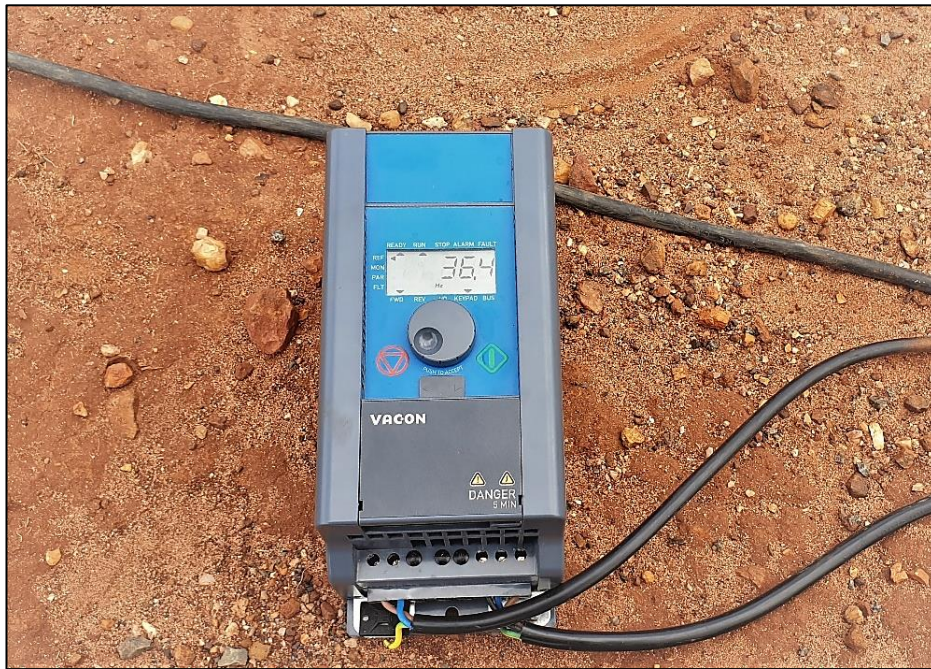
Figure 3.13: Variable Frequency Drive.
