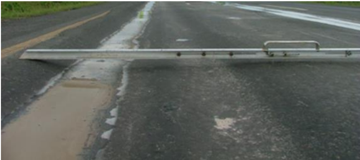
Figure 2.24: Asphalt pavement rutting
