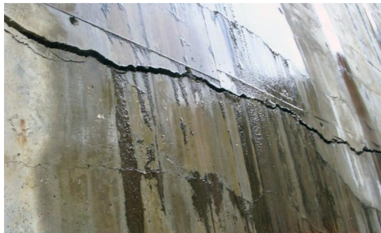
Figure 2.2: Damaged tunnel lining with extensive water leakage
