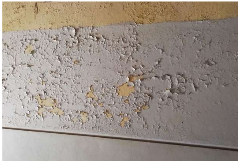
Fig.91: (Left) Surface of the exterior skin of the Capitol theatre: unarticulated and in a state of decay (Author 2021).
