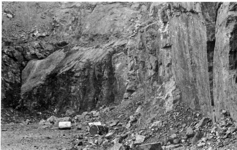
Plate XIV. Thrust shear planes lower the stability of quarry sidewalls when quarry faces are almost parallel to the strike. Note the curving fracture planes at the right of the photograph.
