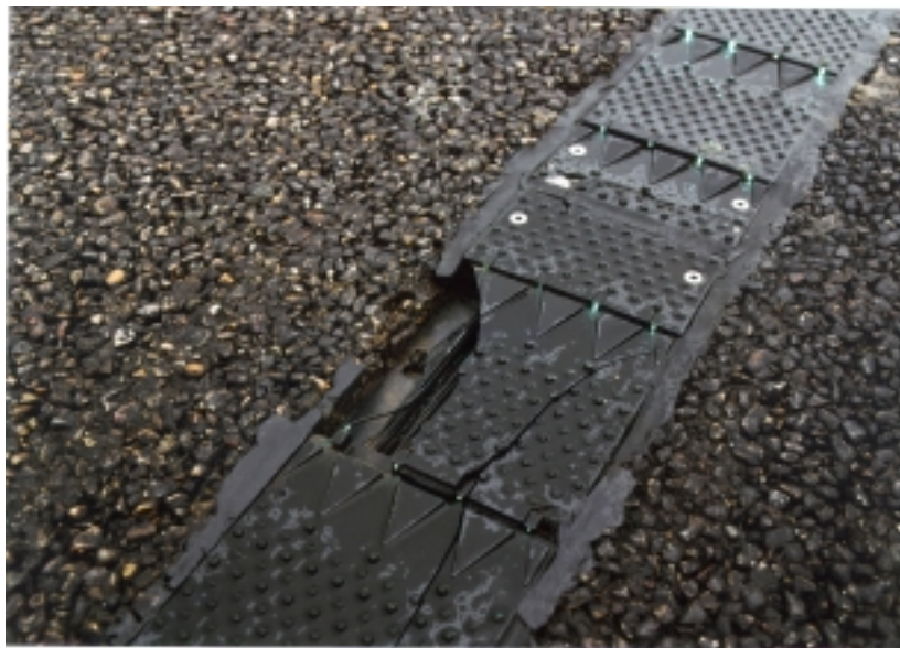
Fig. 6 Damaged part of dynamic road marking
