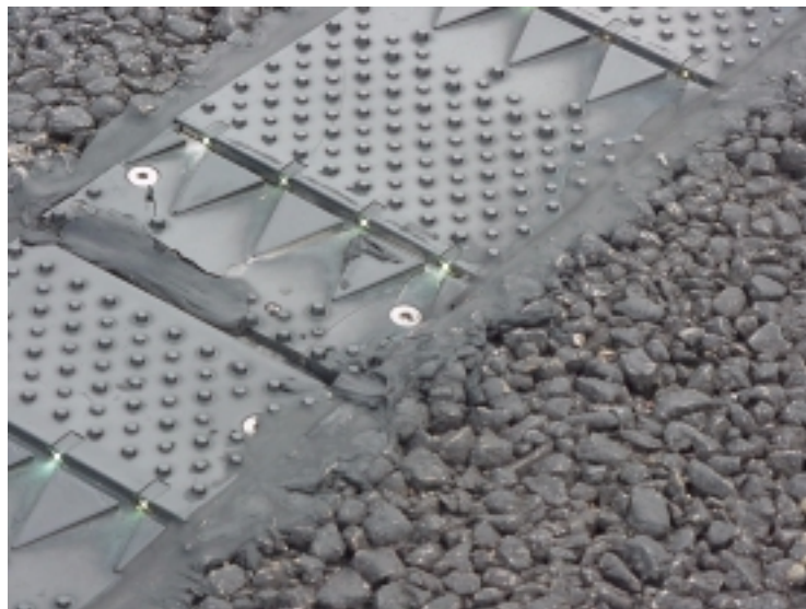
Fig 3. Luminaire of polyurethane containing optical fibres as mounted in porous asphalt
