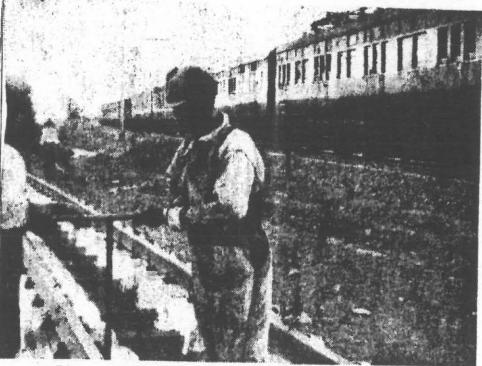
TOP: While a passenger train moves along the threatened Rand-Cape main line at a snail's pace, workers are hurriedly completing a new by-pass line.
