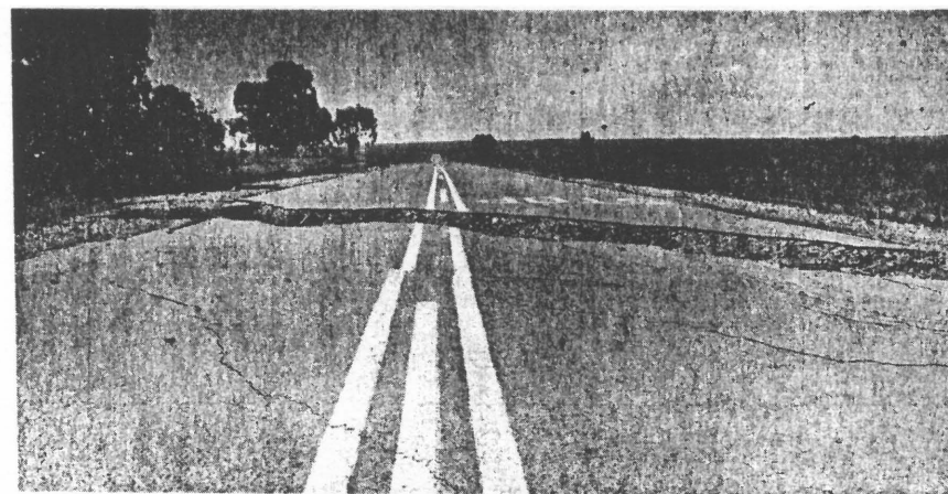
Buckled roads where no car dare cross. The cracks appeared only weeks after Bank became deserted.
