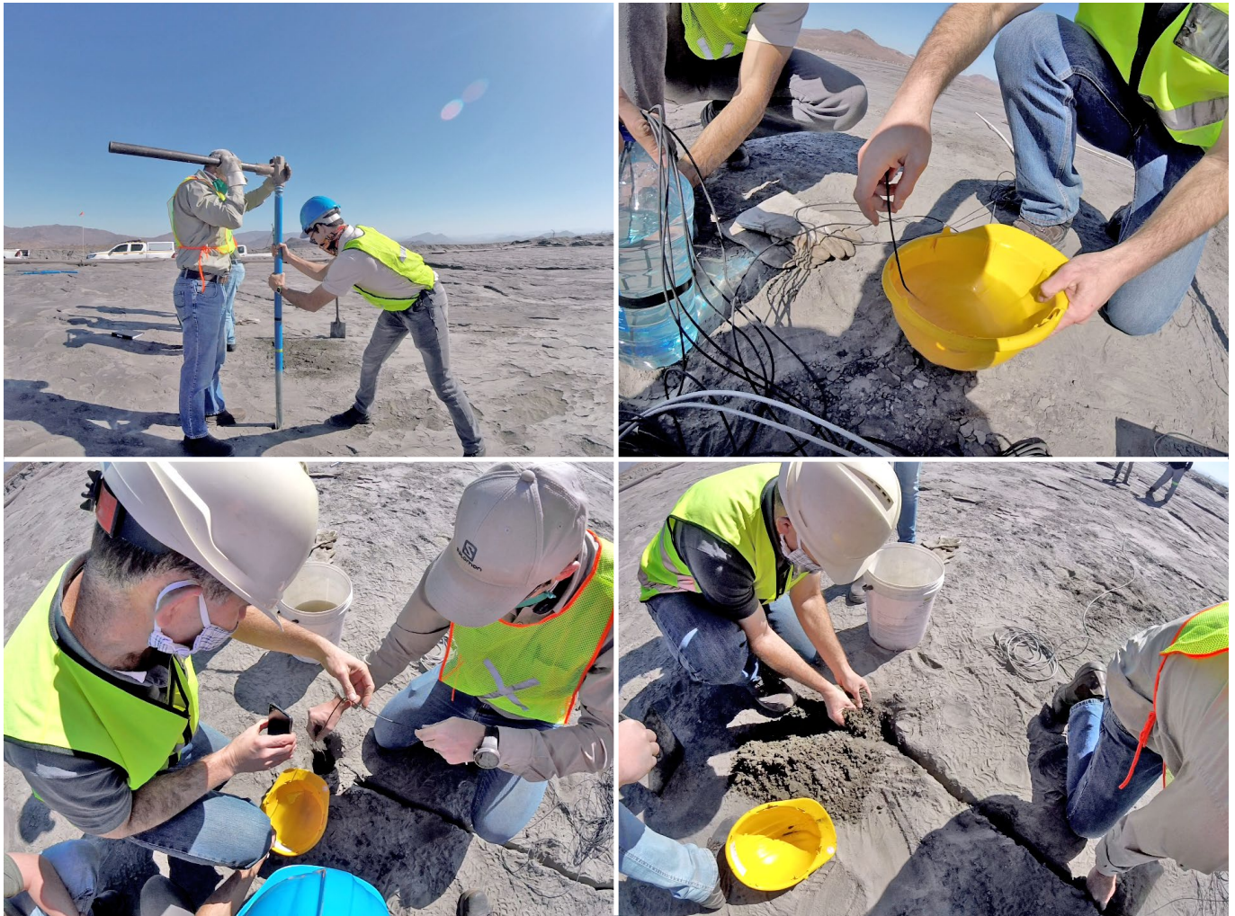
Figure 6 Installation methodology: pole installation (top left), tensiometer transfer from water vessel (top right), installation of tensiometer (bottom left) and backfilling (bottom right)
