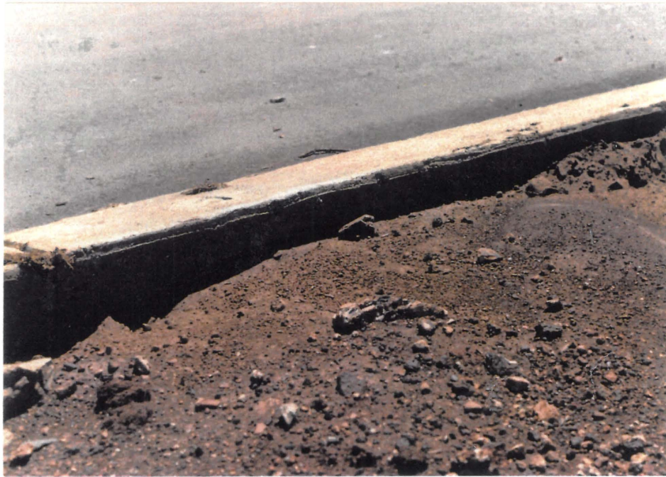
Plate 7: Poor drainage manifest along roadside.
