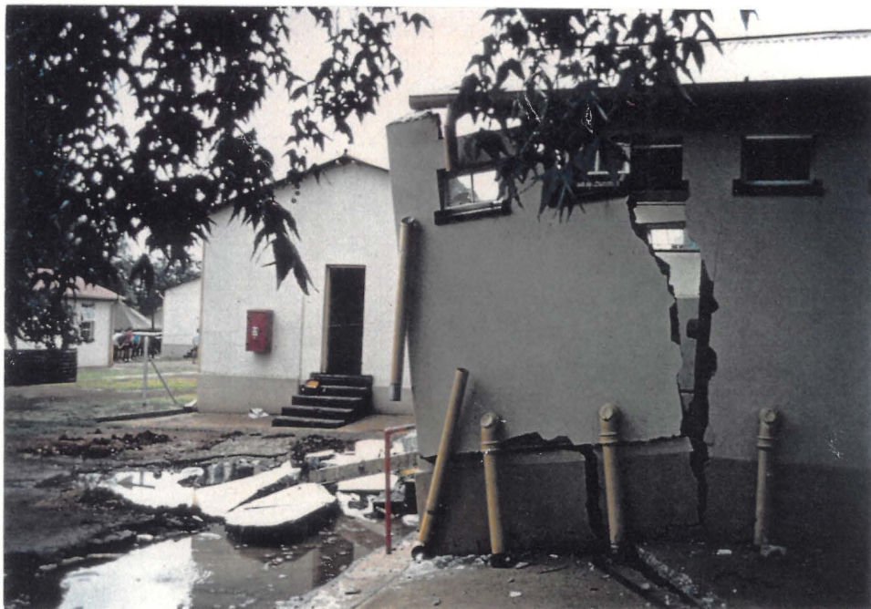
Plate 3: Ablution block in complex south of Pretoria suffering severe structural distress.
