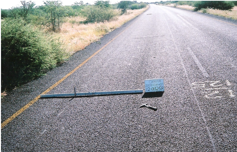
Figure 2: View of Section 12 in Orapa lane after 0,3 MESA in 19 years
