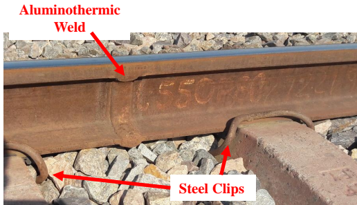
Figure 9: Steel clips in a rail with aluminothermic weld.
