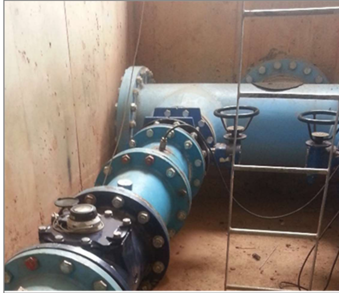
Figure 3-20: AmpAir installation in Pierre van Ryneveld valve chamber (prototype 1)
