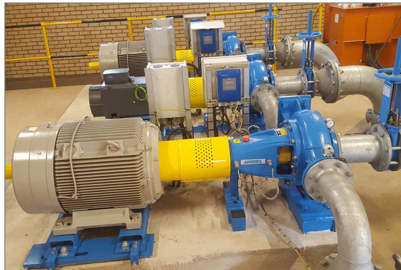
Figure 2-14: Annlin installation – type 1, grid-connected, pumps-as-turbines
