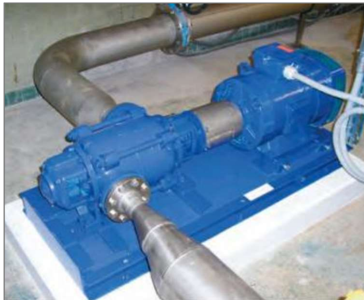
Figure 2-8: A 22 kW Vogel pump turbine in the canton of Friborg, Cornaux
