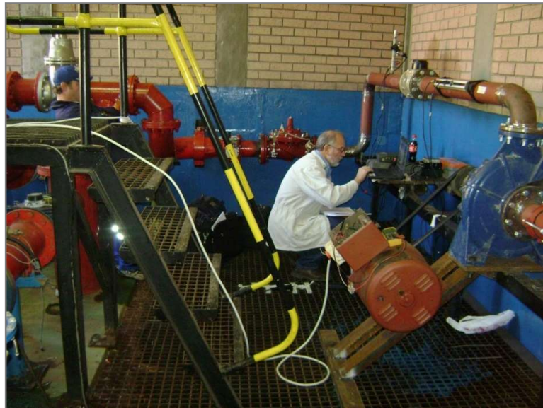
Figure 2-13: Pump-as-turbine testing installation – type 2, first installation
