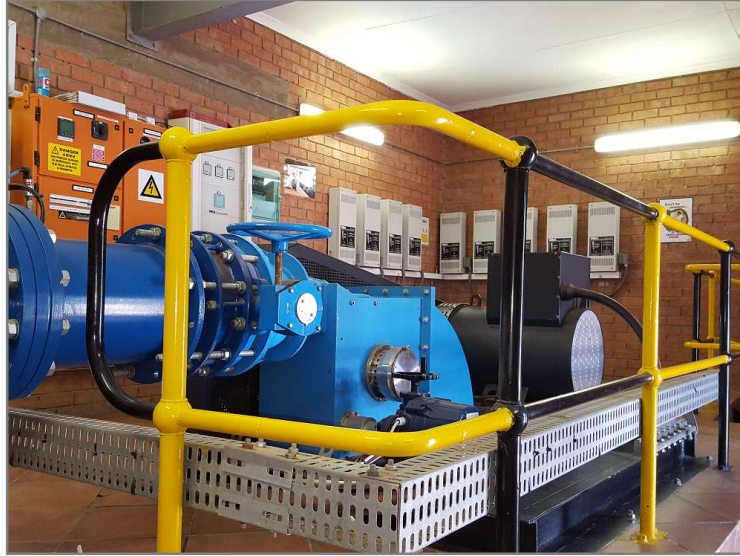
Figure 2-12: Turbine installation at Bloem Water’s Brandkop reservoir. Crossflow (Banki) – type 2, island installation
