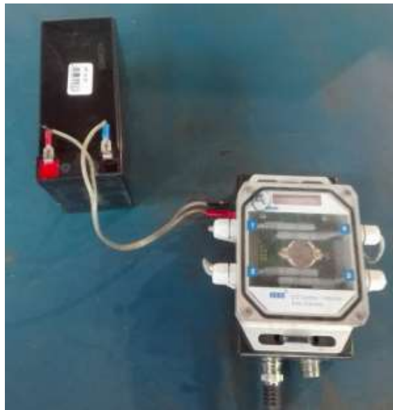
Figure 4-24: The HOBO logger connected to a power supply and pressure transducer
