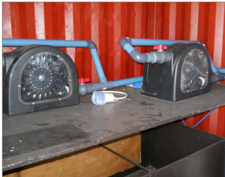
Figure 2-16: eThekweni Municipality Newlands installation, two Pelton turbines – type 2, island installations
