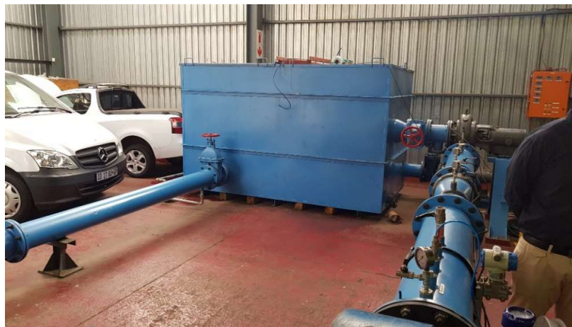
Figure 4-20: A water tank as water supply at the test bench
