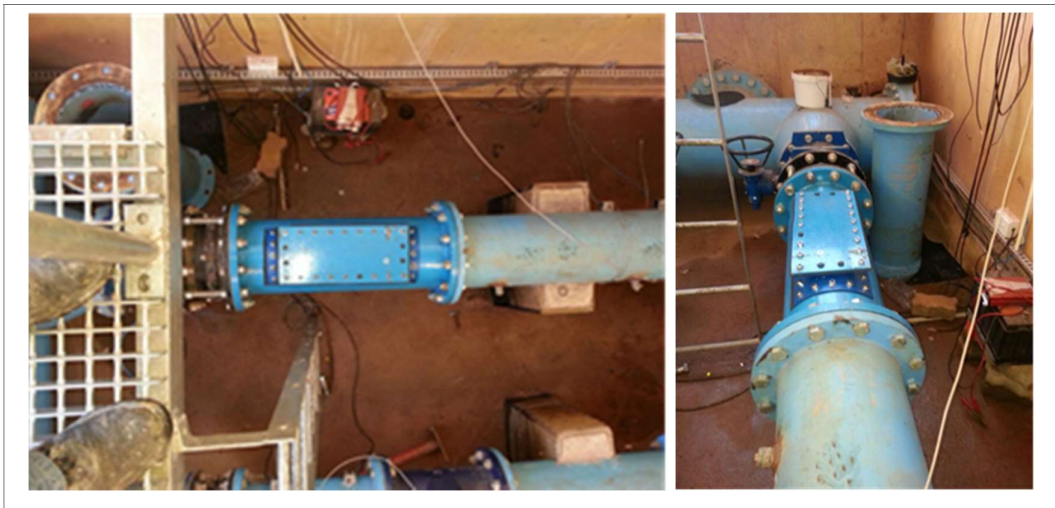
Figure 4-16: Retrofitted mounting piece for an inline pico hydro turbine
