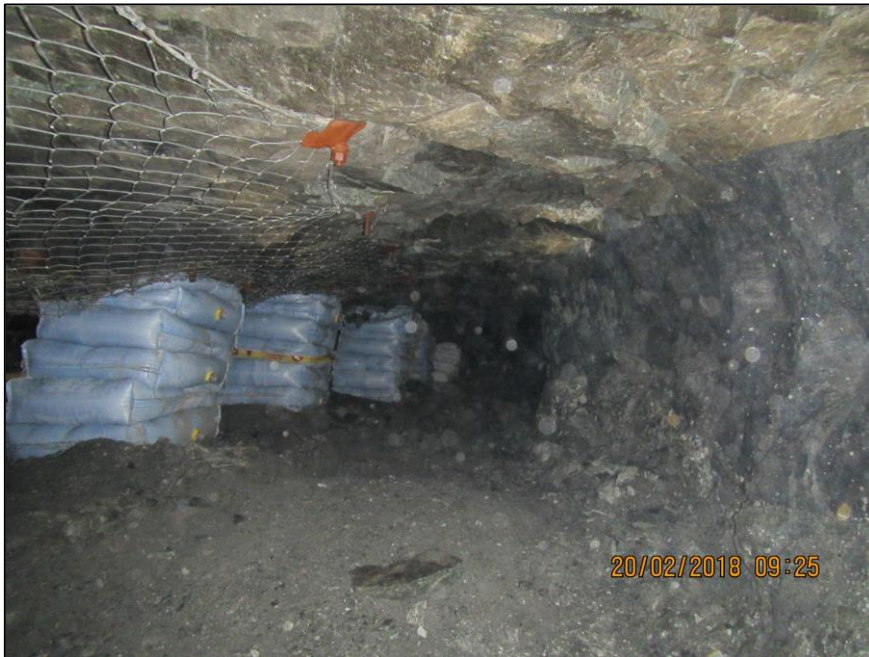
Fig. 2. Use of permanent blast resistant steel nets in the face area of a platinum stope. Visible in the photograph are the other support elements namely rock bolts and cementitious grout packs.
