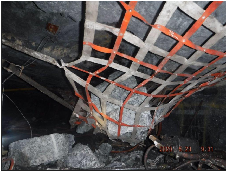
Fig. 1. A fall of ground arrested by a temporary net in the face area of a platinum mine.
