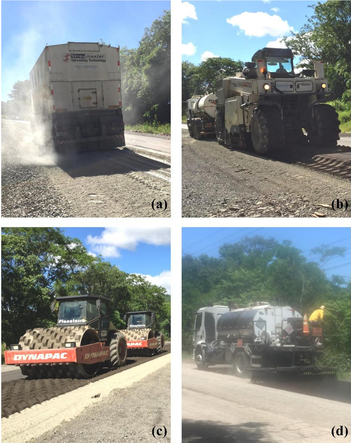
Figure 1. FDR-PC construction: (a) cement spreading; (b) pulverisation/mixing; (c) compaction; and (d) curing membrane application
