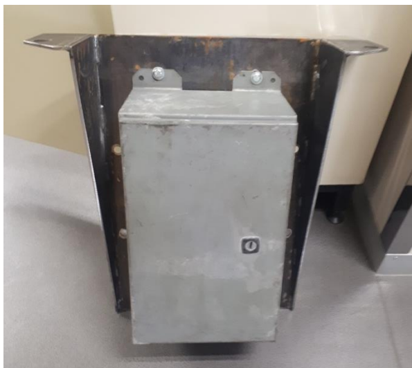
Figure 83 Manufactured mounting bracket and equipment enclosure
