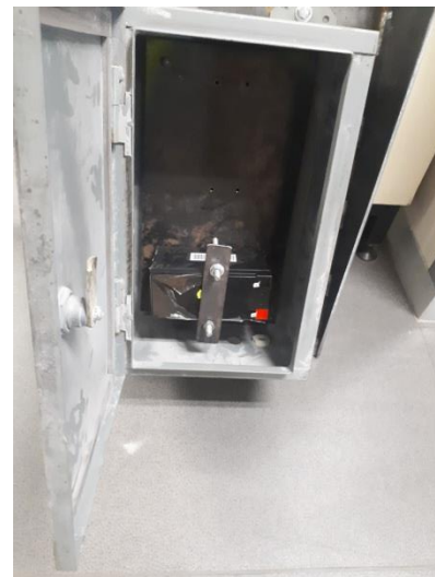
Figure 84 Inside equipment box, manufactured backing plate and battery visible
