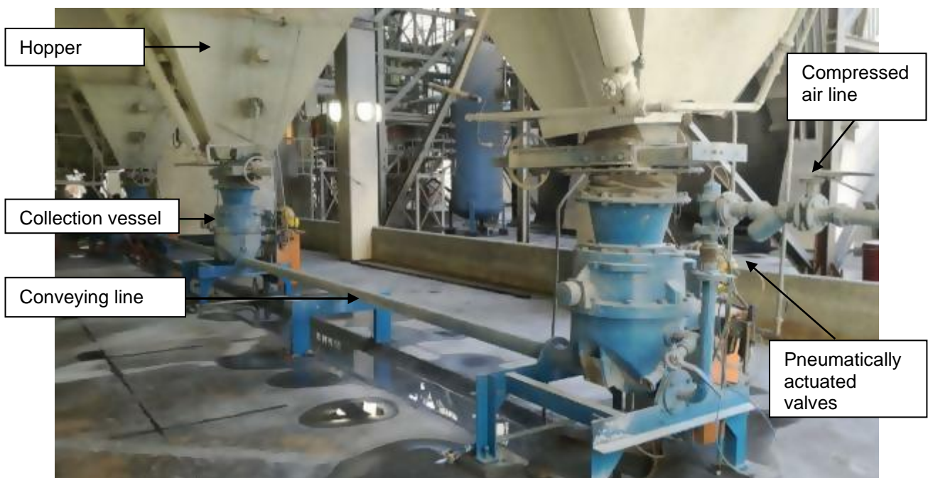
Figure 1: Pneumatic conveying plant
