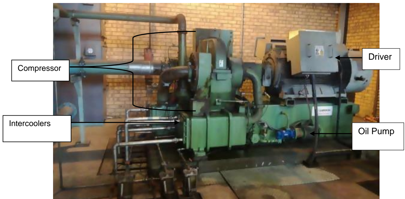
Figure 2: TA-3000 Integrally geared centrifugal compressor (Courtesy of Kriel Power Station)
