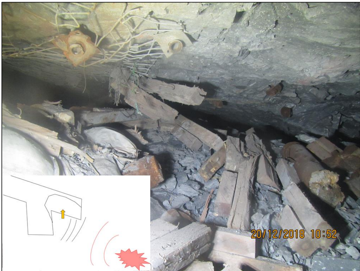
Figure 35. Footwall heave in south siding.
