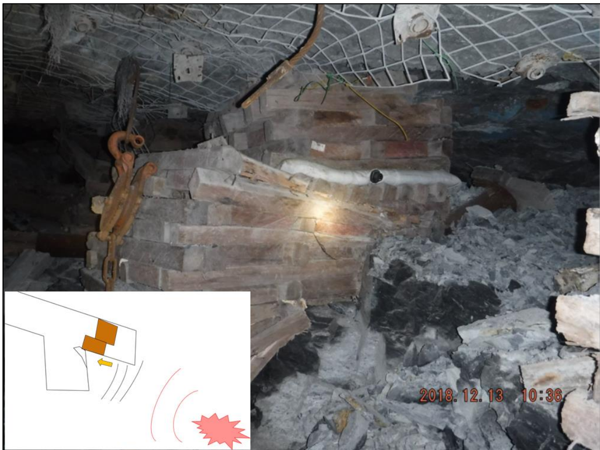
Figure 34. Siding sidewall (southern) movement and pack shear.
