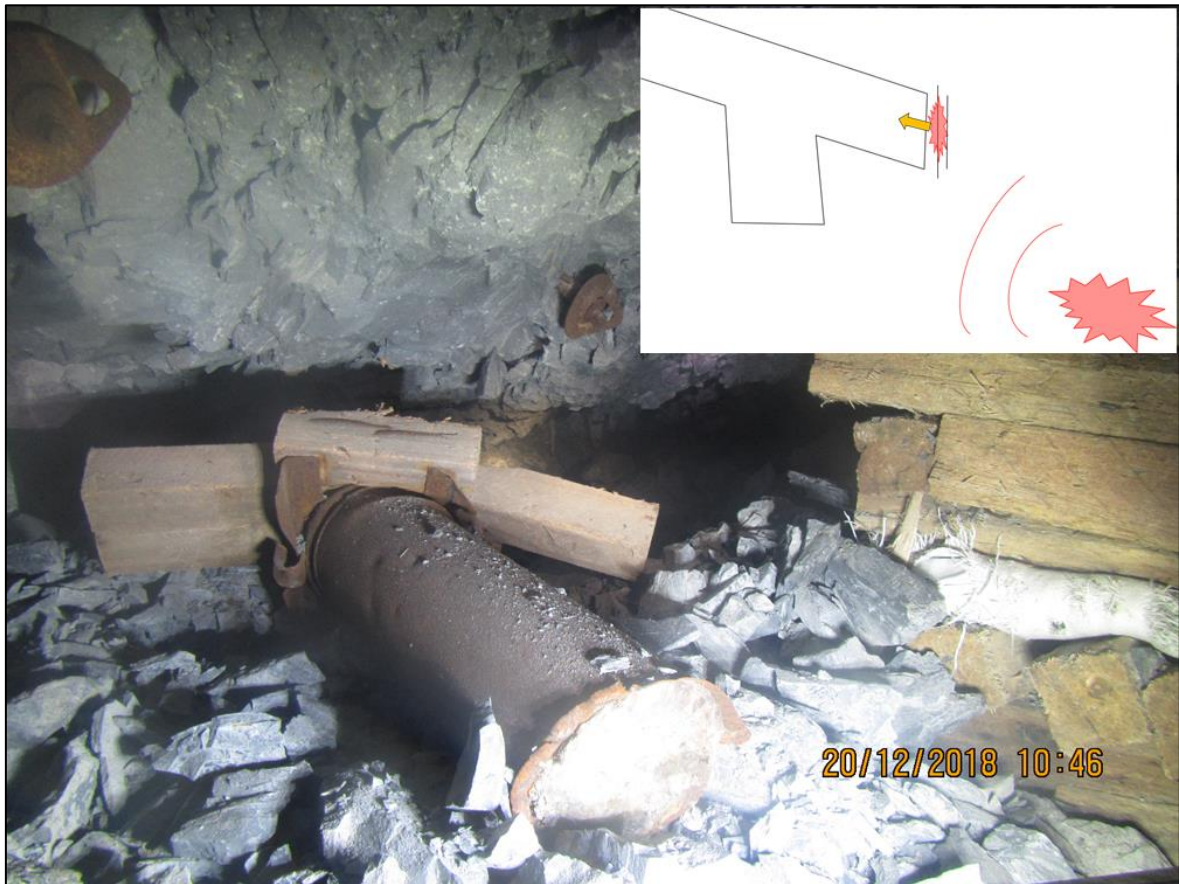
Figure 33. Observed ejection from south siding abutment.
