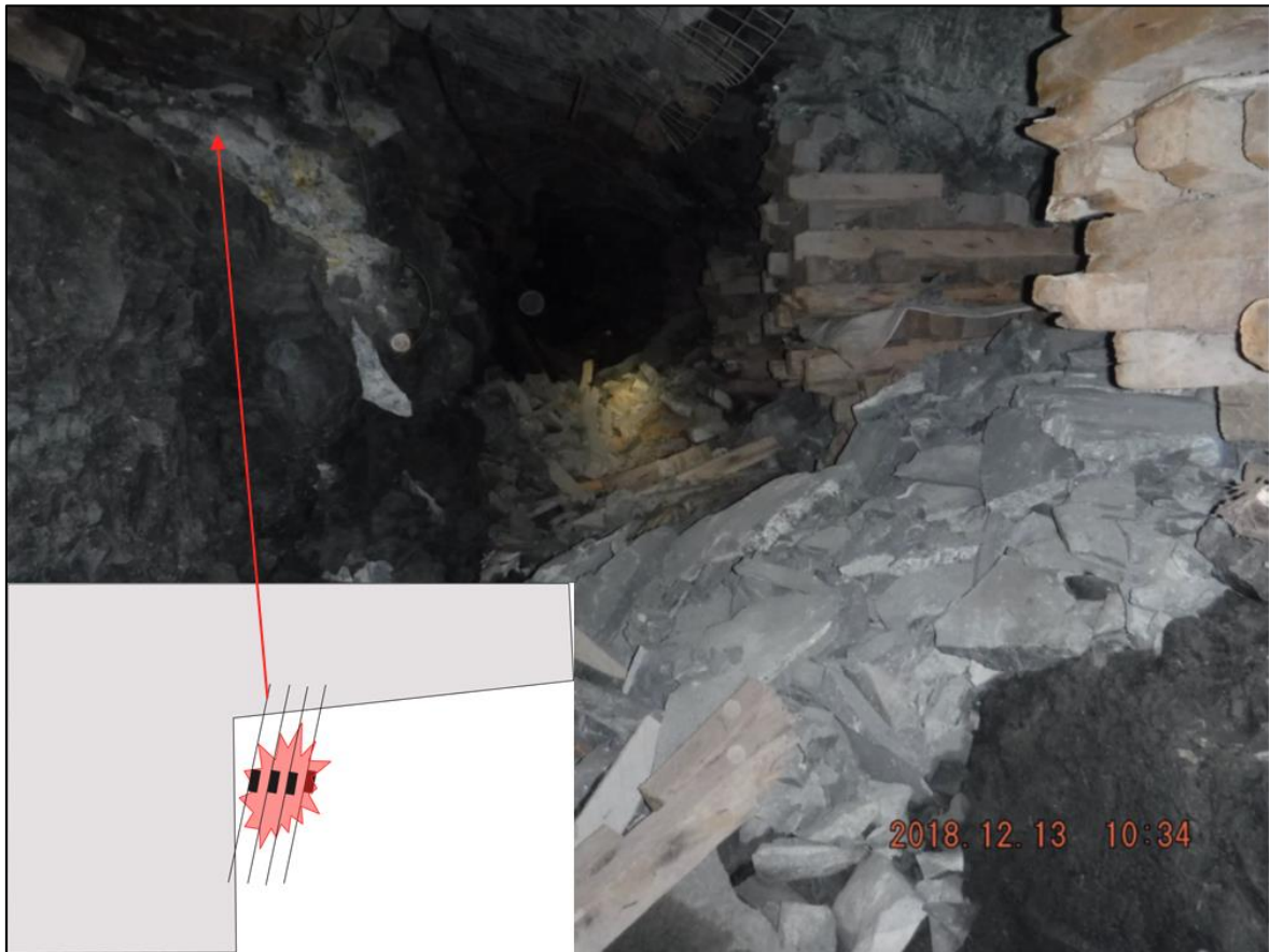
Figure 31. Shear zone observed in gully northern sidewall and stope footwall.
