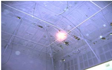
Fig. 2.9: The only vaulted pressed steel ceiling in the building, painted purple (Photographs by Niebhur (2008))
