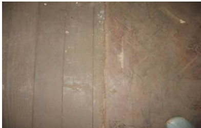
Fig. 2.8: The original 'Oregon Pine' timber floor was later covered with a layer of parquet flooring (Photographs by Niebhur (2008))
