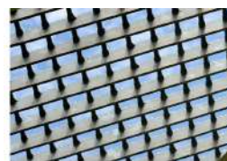
Fig 8.19: Mentis grille For the green house to allow movement of air and for storm water covers to allow catchment of debris
