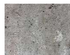
Fig 8.20: Concrete floor slab for flooring to allow robustness and durable to wear and tear
