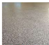
Fig 8.18: Epoxy floor finish Epoxy flooring finish applied to hard wearing surfaces in public areas for ease of maintainance and cleaning
