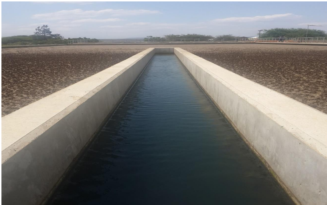
Figure 21: Plant 3 sedimentation tank overflow weir, bulking sludge and accumulated suspended solids on the surface.
