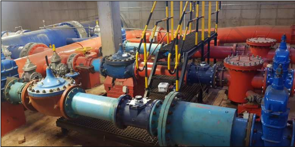
Figure 5: PRS located at the inlet to the Salvokop reservoir (Pretoria, South Africa) (Color)
