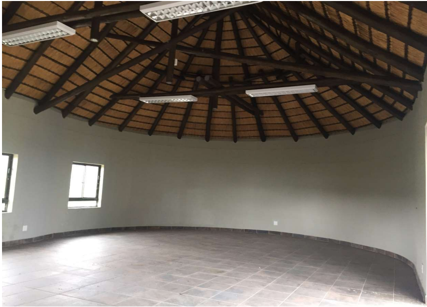
Fig. 17: A large open area inside the tourism centre which will probably be used to showcase images of the rock art and provide tourists with more information about the surrounding area.
