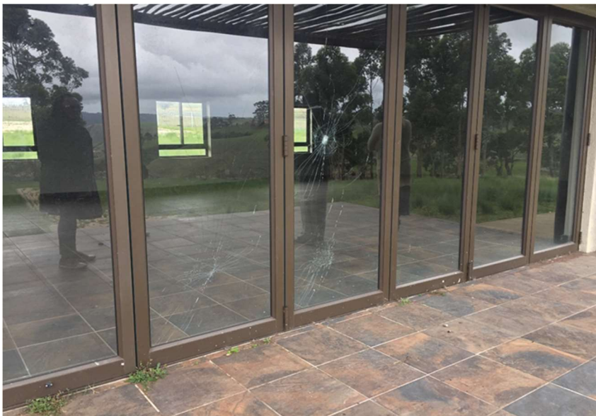
Fig. 13: The large glass doors in the back of the tourism centre. Some panels have been damaged by what looks like a large stone or brick thrown against it.
