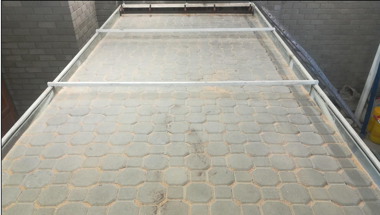
Fig. B-5: An image showing the completed construction of a Citylock® and P-Type 1 sand containing layer works in the Full-scale Model shortly before testing.
