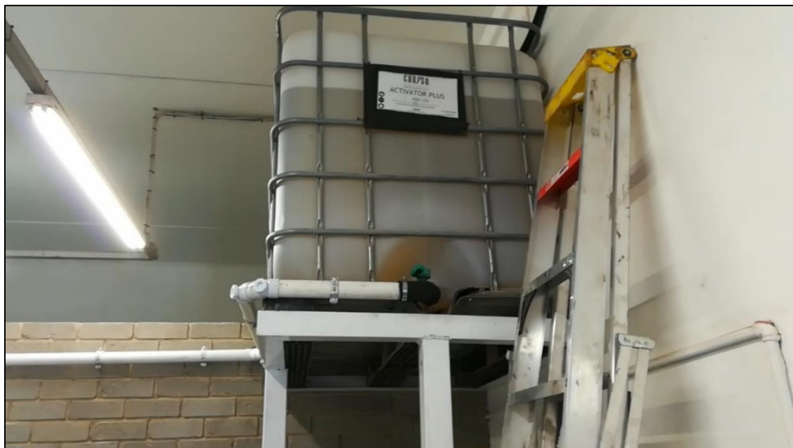
Fig. 13: The 1000 ℓ water tank that provided water to the ITA for testing (Bosun – Midrand, 2018).
