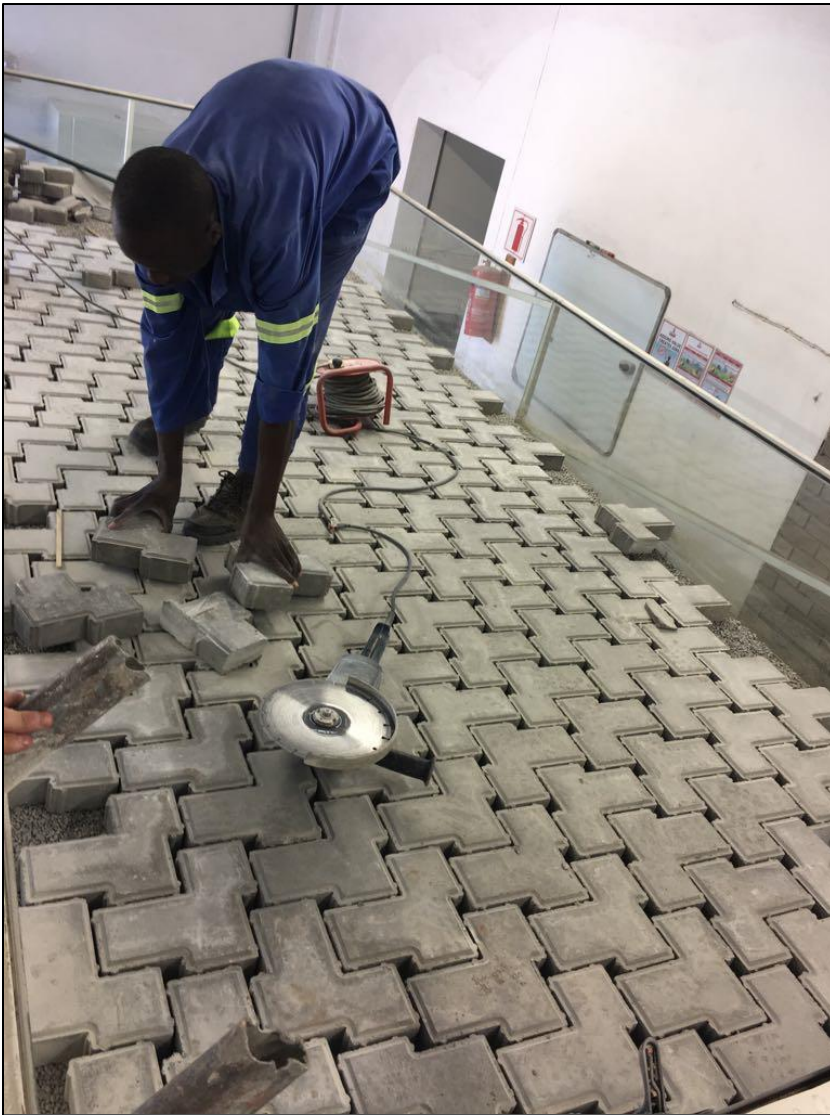
Fig. B-3: An image of the way the Waterwise® concrete bricks were laid during construction of the Full-scale Model layer works.
