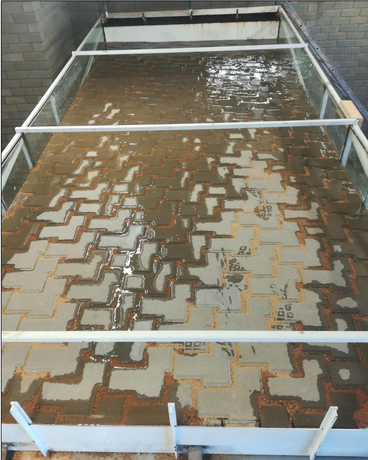
Fig. B-7: An image showing the testing of a Waterwise® and P-Type 5 sand containing layer works during the Model Design testing. Here, the wetting front can be seen traversing the full length of the pavement.
