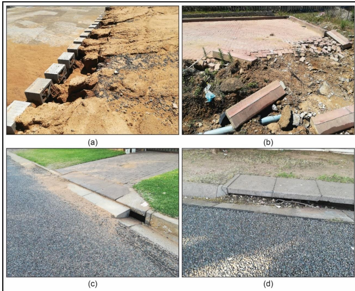
Fig. 1: An example of erosional damage to a retaining wall (a), damage to an interlocking pavement due to poor drainage (b) and two stormwater drains clogged by silts and organic matter (c) and (d) in Gauteng province respectively.
