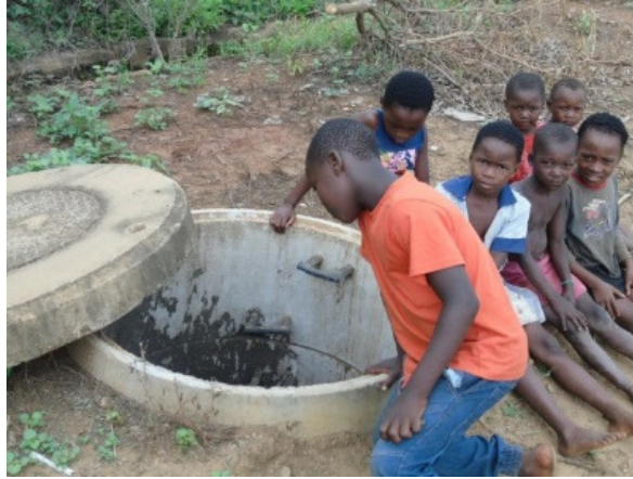
Photo 22: An indication of poor management at sewer system infrastructures in Pongola. Children are playing around an open sewer mainline manhole.
