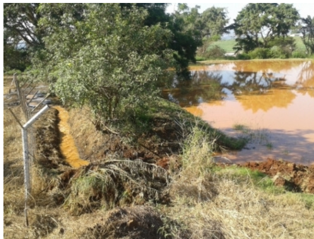
Photo 21: An indication of poor management at the potable Water Treatment Plant in Pongola. During the severe 2015 drought, the plant manager decided to dig trenches alongside the water reservoirs to release excess water from the holding reservoir instead of closing the inlet sluices.
