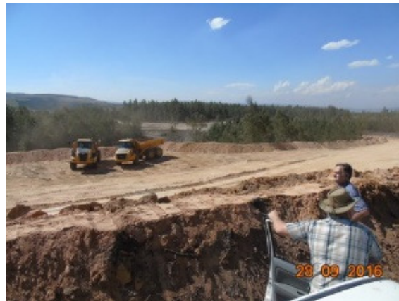
Photo 10: Open cast excavation of a coal mine that obtained a mining permit without a proper procedure and without the knowledge of interested and affected people in the area.
