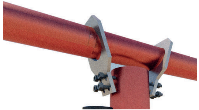
Figure-163: Step 2- Fixing the structural round tubing spine to columns with the custom brackets.
